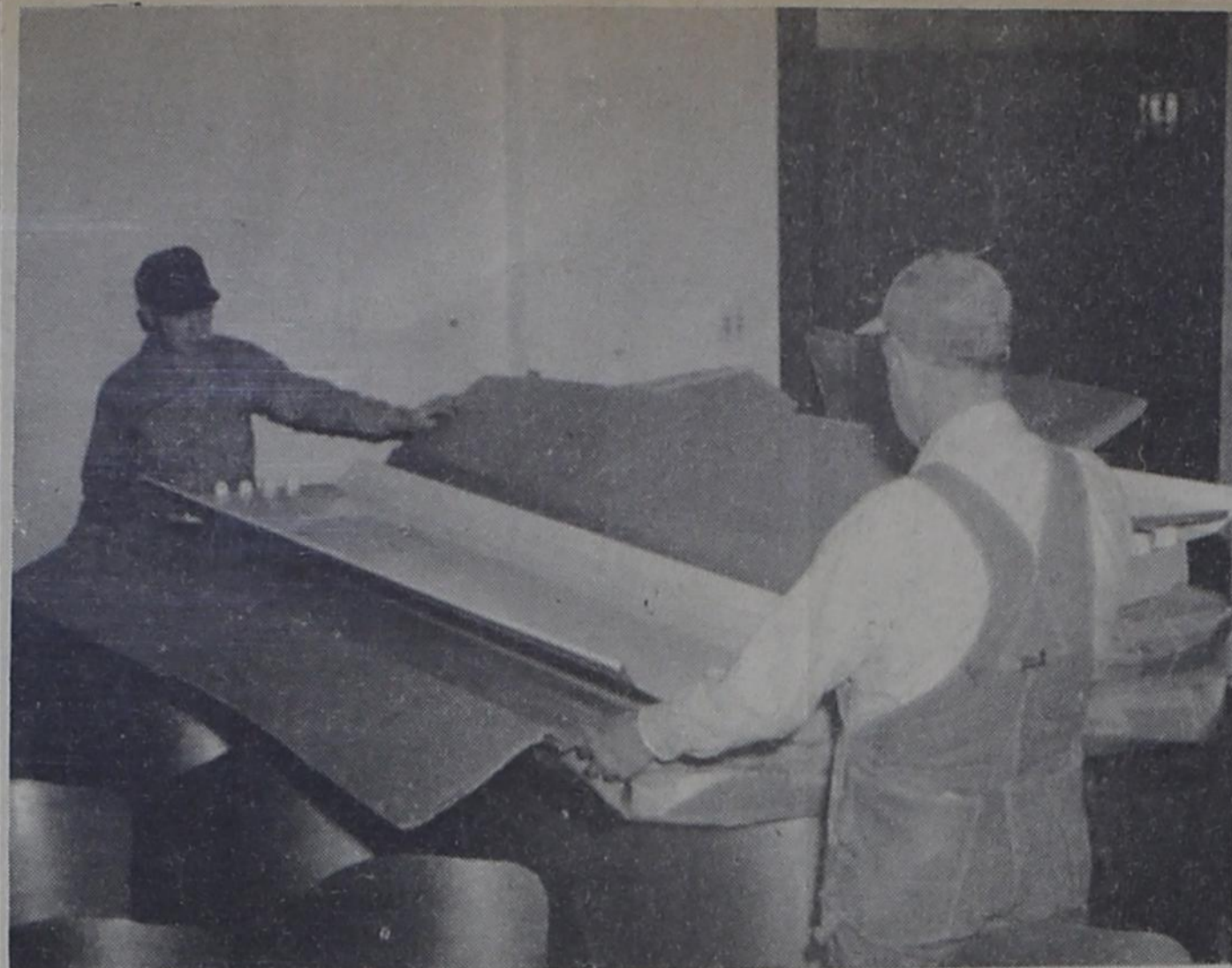
A NEW FACELIFTING for the district courtroom on the second floor of the Parmer County courthouse was in progress this week. Here, workmen unbox fluorescent fixtures for the new lighting system. The balcony is being eliminated, and the ceiling lowered several feet. Acoustical materials are expected to improve considerably the ability of those in the courtroom to hear one another.
