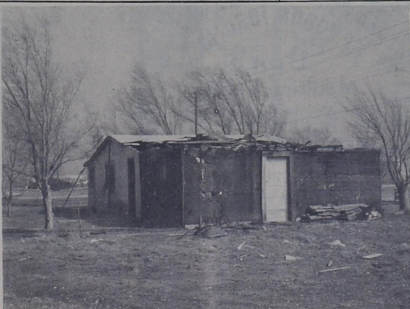
WIND DAMAGE -- High winds accompanied by blowing sand took their toll in Bovina Friday. A large portion of the roof on the house of Mr. and Mrs. Paul Gonzales was torn away by the high winds and deposited in the middle of Fourth Street. Wires, antennas, etc. over town also received their share of damage.
