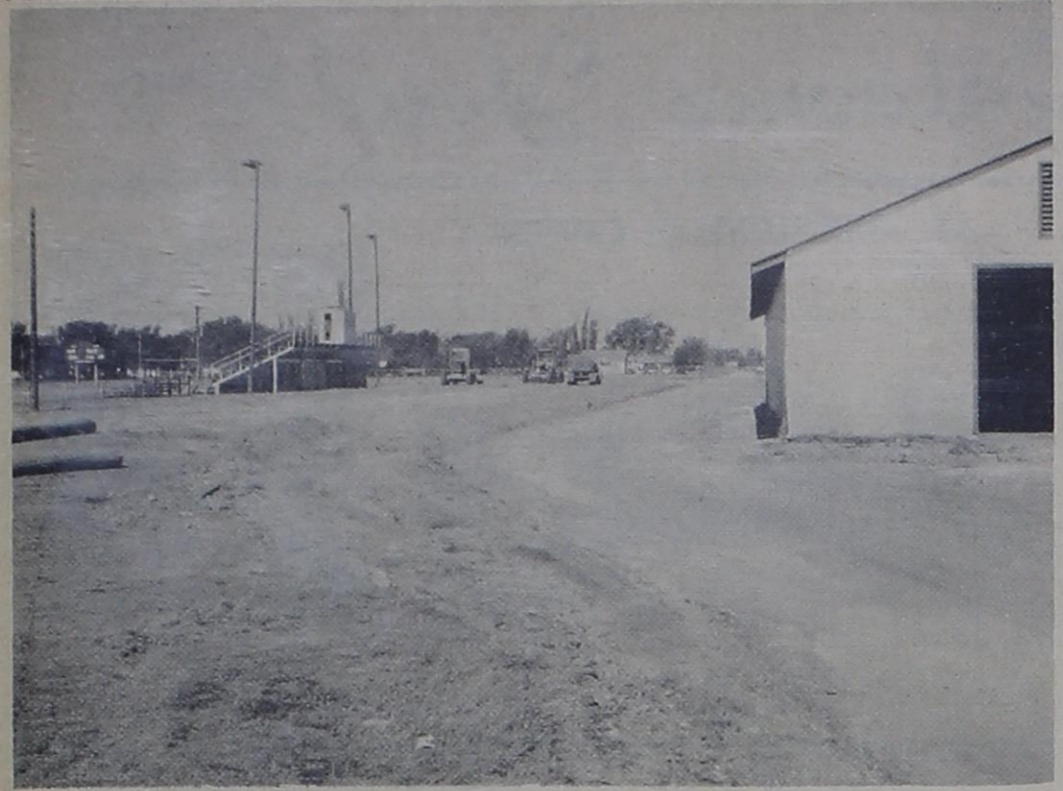
SCHOOL IMPROVEMENTS -- Paving of the street between the football field and the Bovina Schools, as well as the parking area behind the football field, got underway last week. The unpaved street had become a problem for loading and unloading bus students. Jake Diel, who is contractor for city paving, was awarded the contract at the school for $1.55 per square yard.
