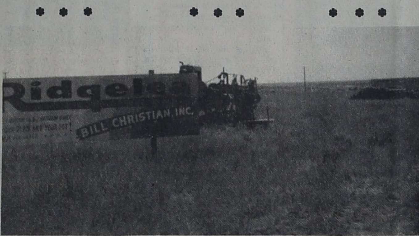
ACTIVITY--Final details for installation of water and sewer lines in Ridgelea, Bovina's proposed housing development, were ironed out Monday work began. A ditchdigger is shown at right of Ridgelea sign and at far right are stacks of pipe which will be used.
