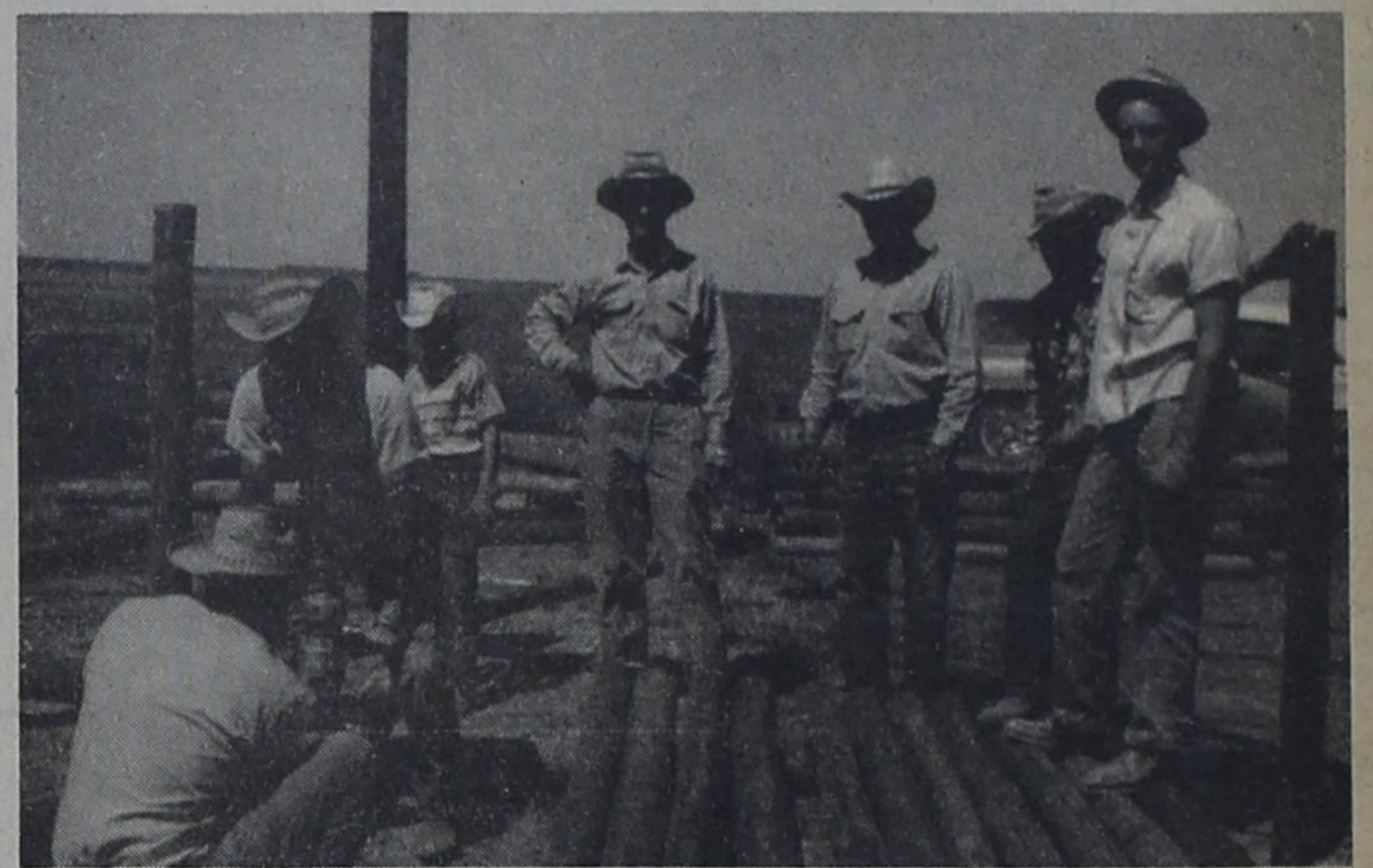
FENCE BUILDERS--Friday was work day for members of Bovina Rodeo and Roping Club at new arena they are building west and south of town. The arena is scheduled to be complete late this summer and ready for use by next spring. Posing for camera here, from left, are Tiny Walling, back to camera; Marion Carson, with bit; Alan Carson, R. T. Harbour, Rouel Barron, Robert Galaway, and Robert Read.
