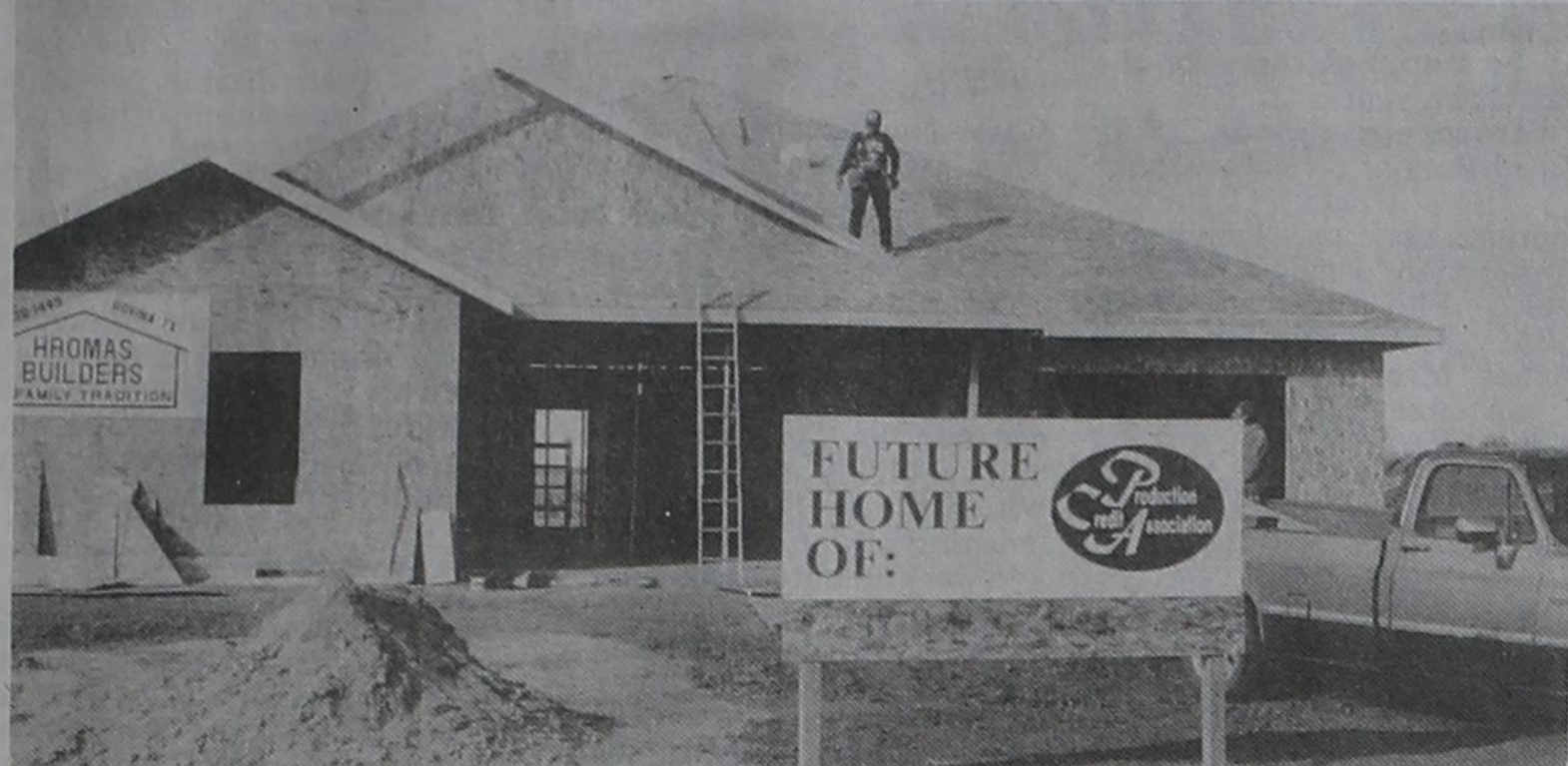
A NEW OFFICE building on Highway 60 in west Friona will house Production Credit Association. The new offices are near Headquarters Restaurant and are being built by Hromas Builders of Bovina. Owner Galen Hromas is Bovina's mayor. ron carr photo
