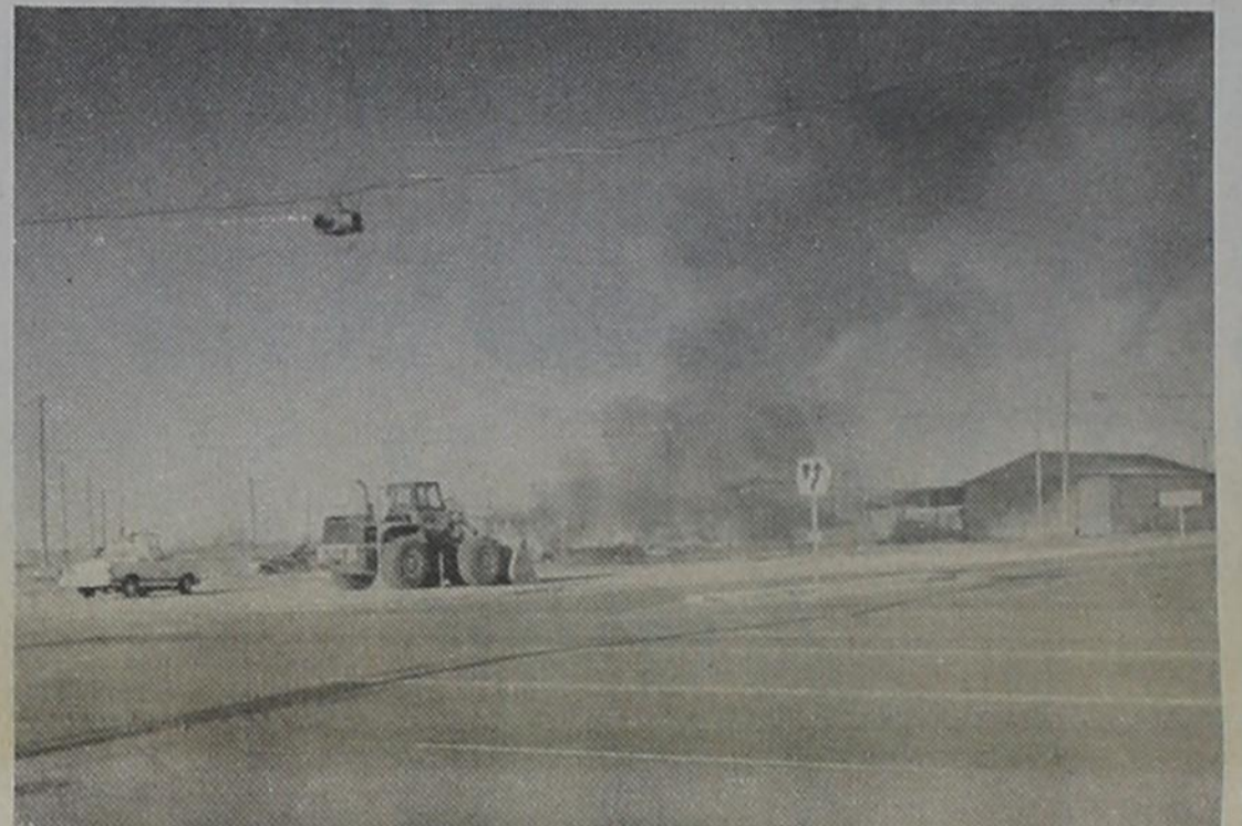
UP IN SMOKE...The old vegetable shed on Highway 60 was demolished and burned this week in the city's continuing program to get rid of old, unsafe buildings.
