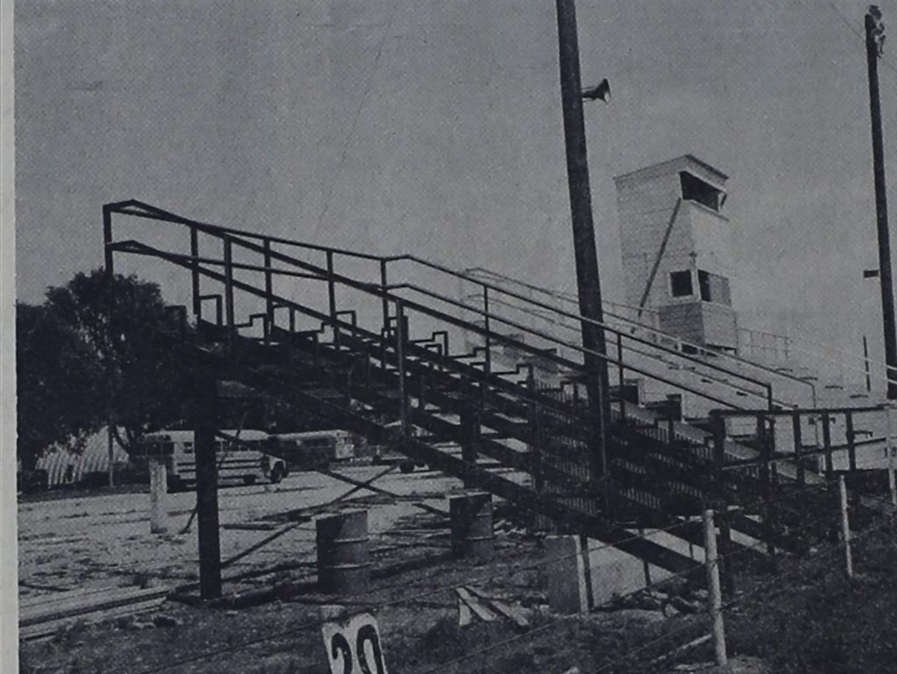
NEW SEATING ADDITION --- Construction work is nearing completion on a new 20-foot section of bleachers at Mustang Field. The additional stands, designed to seat 180 people, are on the north end of the "home" side of the field. Metal work was done by Kerby Welding Service and Sherrill Lumber Co. is in charge of the wood and concrete portion of the stands.
