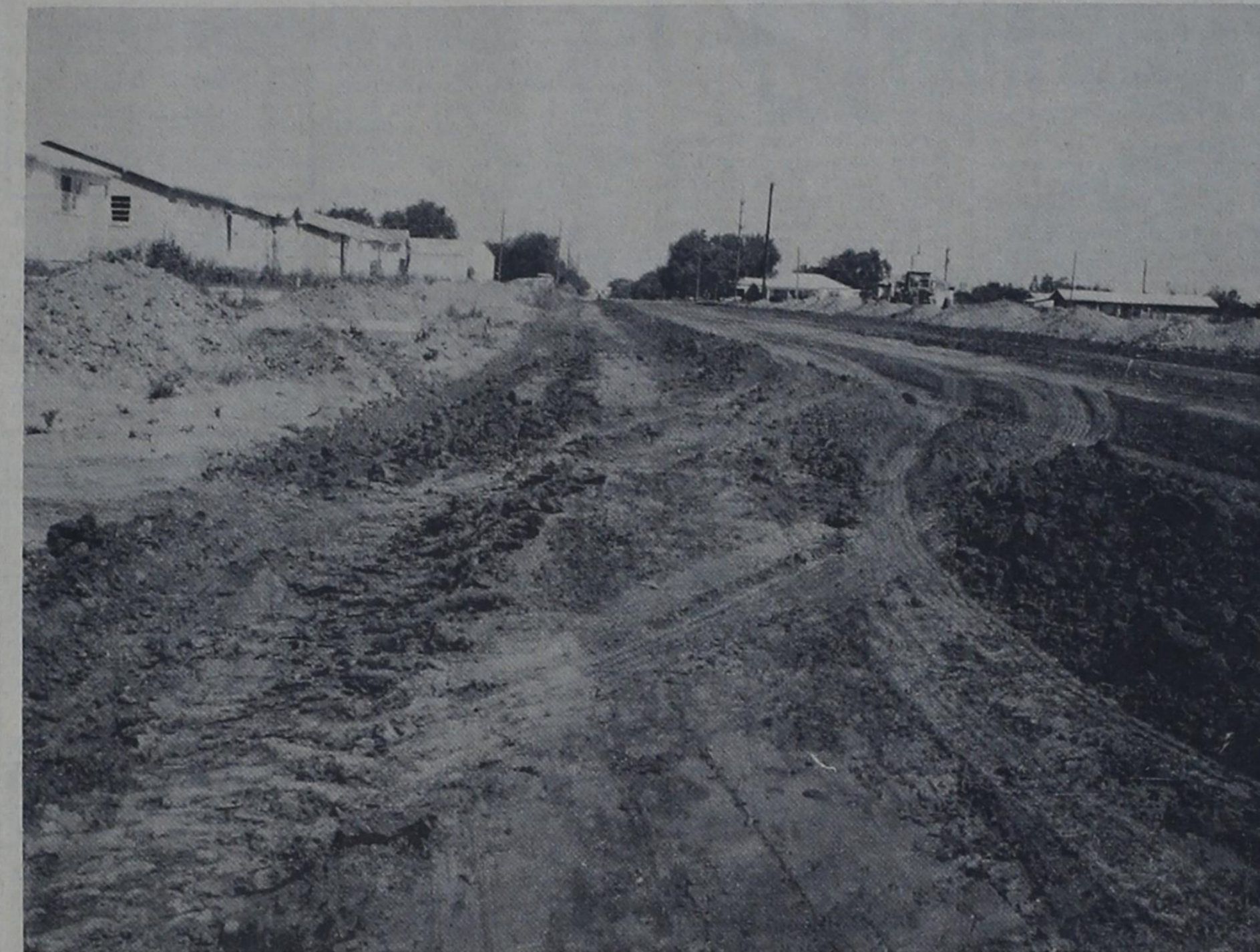
STREET IMPROVEMENT --- Grader work was started last week on Bovina's newest paving project. Curbs and gutters are scheduled to be poured in the next few days with the paving to follow
