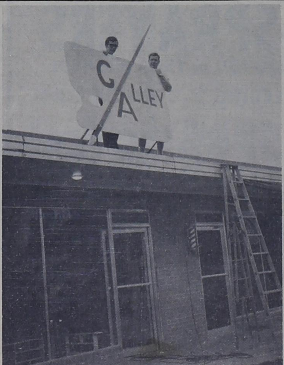
GETTING IT STRAIGHT --- Billy Whitecotton and Jerry Wright check with an observer below to be sure the new sign for Galley Alley is straight. Grand Opening for the art center was held Sunday afternoon.
