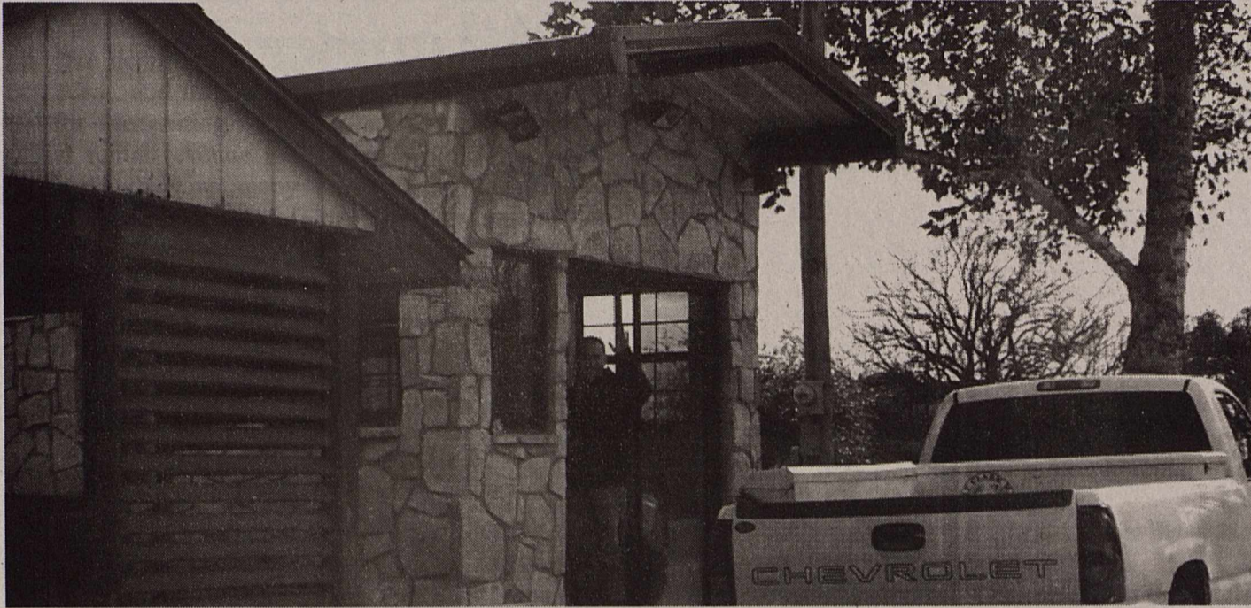
Brackett News Weekly Photo By Leigh Jenkins - Fort Clark Security employee Jose Vela waves on a member from the newly constructed guard shack. The old guard shack at the left is in the process of being torn down.
