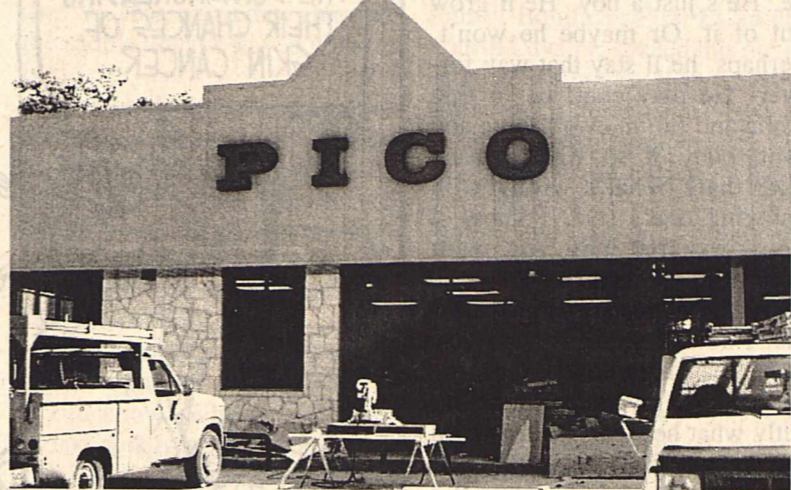
Contractors are putting the finishing touches on the new Pico store which will be opening soon.
