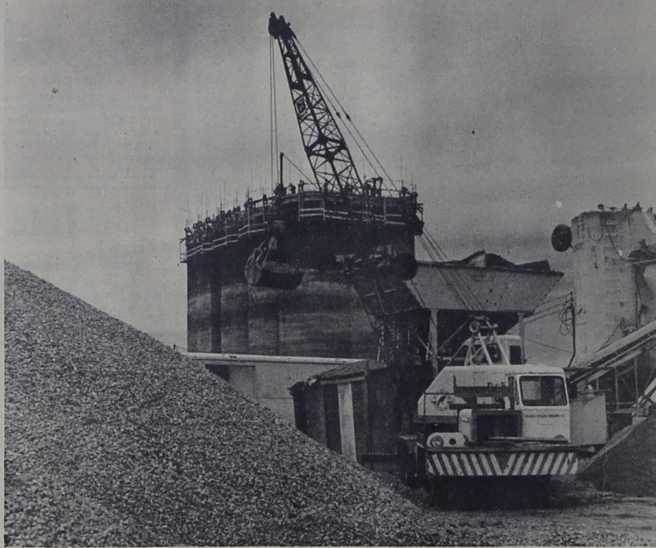
First of its kind--a concrete elevator located some distance from a railroad--is being constructed at Lazbuddie by Sherley-Anderson Grain Co. The one-half million bushel structure is expected to be ready for operation by June 1.
