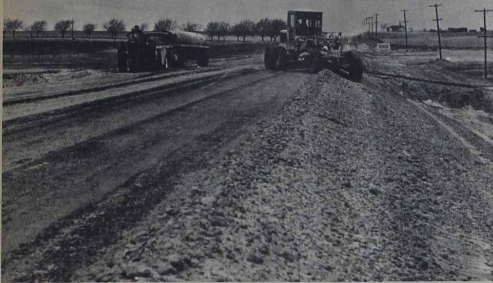
Finishing touches are being applied to a 10 foot fill in the Farmer County end of the paving addition to FM 145 between Lazbuddie and Castro County. Work on the extension of the
