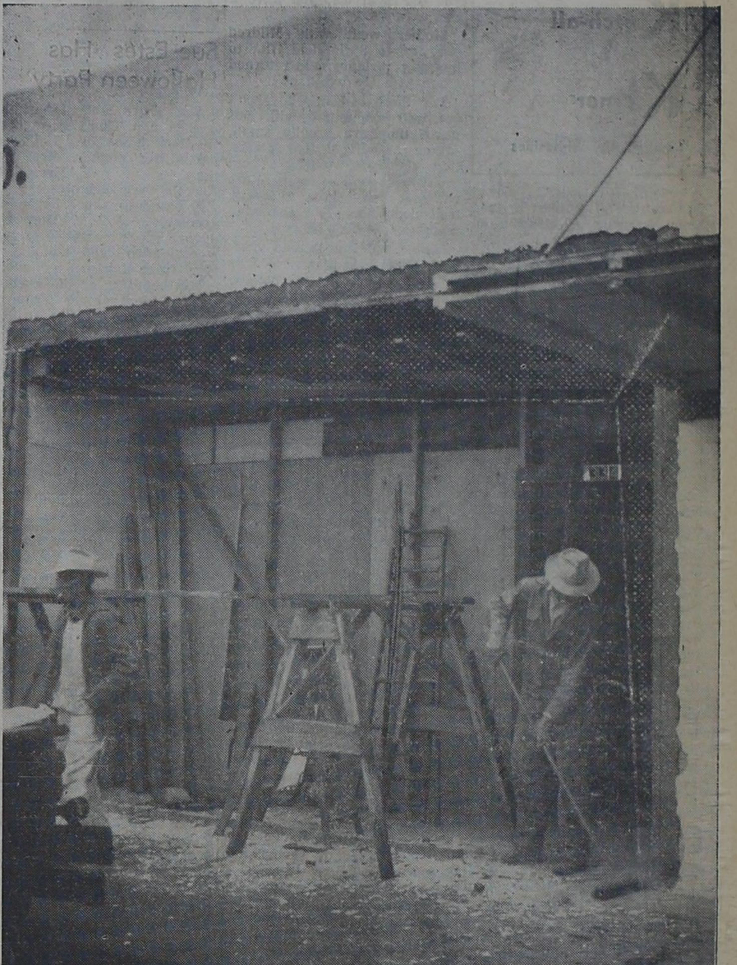
TO REPLACE YOU HAVE TO TEAR DOWN—With everything but details complete on the inside, the remodeling of Bovina's post office had advanced to the point of the building Monday afternoon when this picture was made. Hubert Ellison, contractor, is at right. S. A. Brito, carpenter, is shown walking out of the picture at the left. The remodeling work, which will modernize the post office as well as make for more room, was started some 10 days ago and is scheduled for completion this week.
