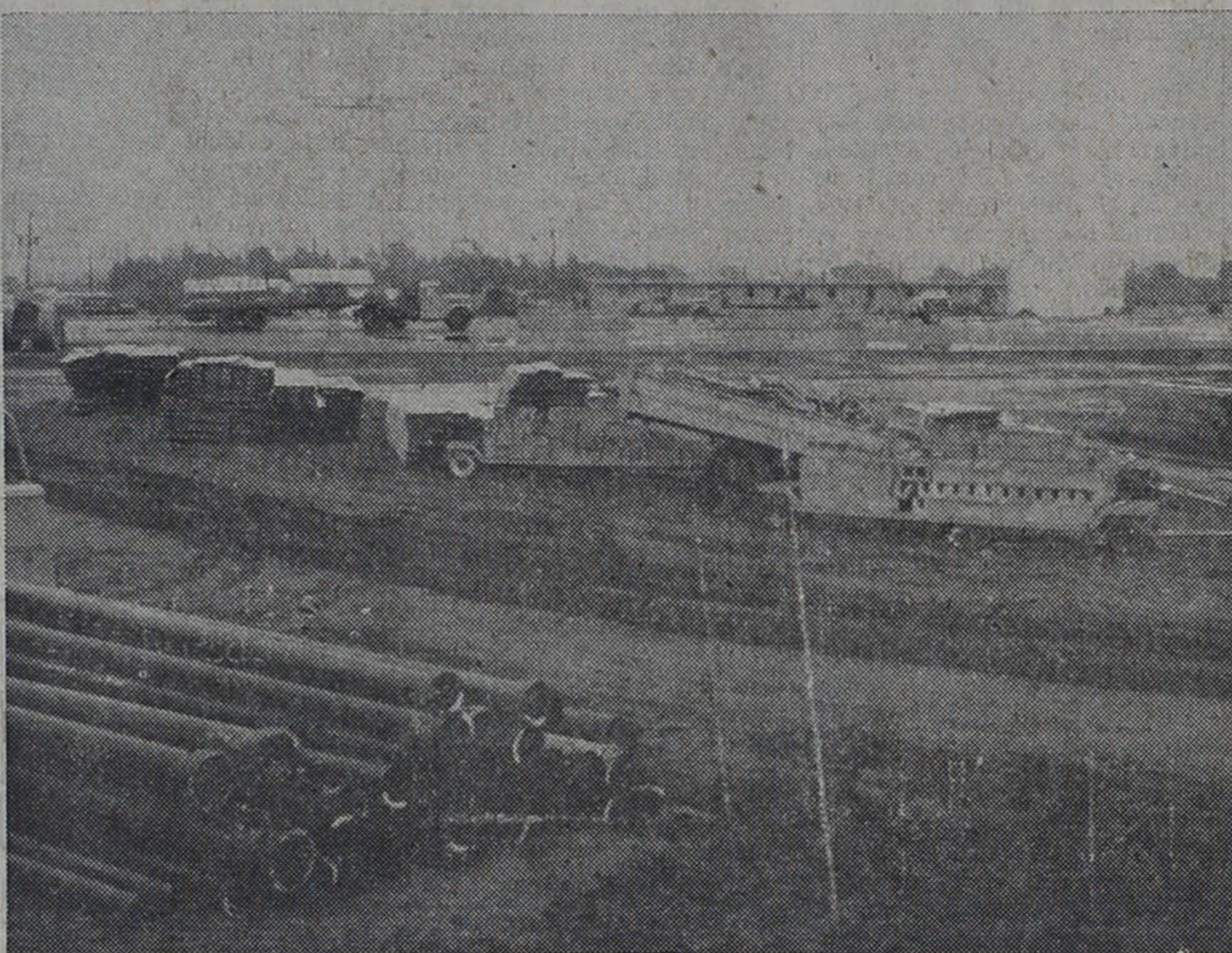
Things are busy at the construction site of Western Warehouse, a cotton storage company, in Bovina. This is the first cotton storage firm to do business in Parmer County, and they began receiving cotton last week. Weather has hampered construction progress.
