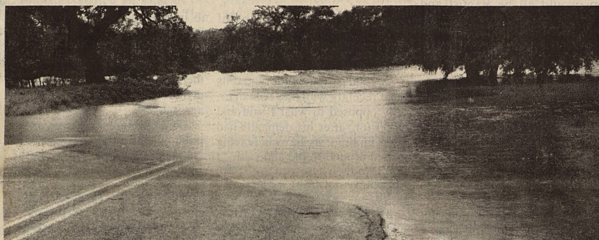
Water flows across the Pinto Creek bridge on R.R. 2804 after rains soaked Kinney County earlier this week. Brackett News Photo by Jewel Robinson
