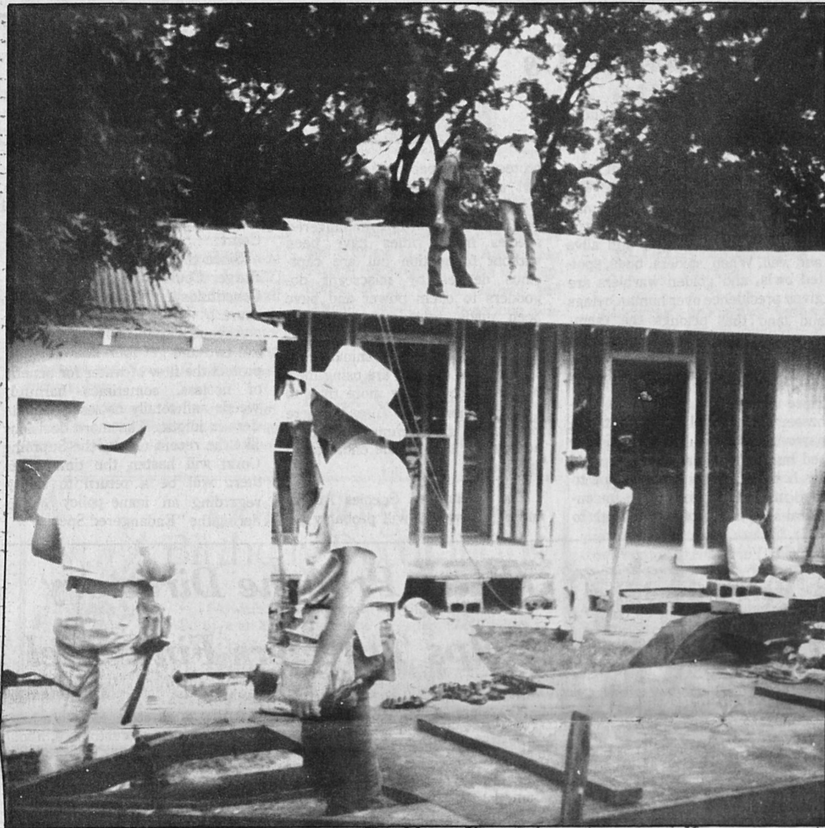
Pictured left to right on the ground are Rick Davis, Sam Snyder, Mike Fielding and Geoffrey Snyder. Left to right on the roof are Dinty Bowman and Billy Boland.
