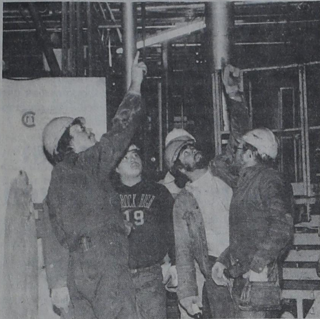
INSPECTING DAMAGE.... Excel workmen are shown inspecting the area which sustained an electrical explosion early Thursday, shutting the plant down for most of the day. Operation at the beef packing plant was expected to be back to normal by this weekend.
