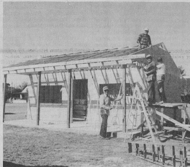
On roof - Ken Callnan; on ground - Jaques Zell; on scaffold - Newell Mayberry and Ron Buckles.
