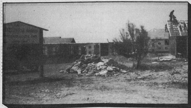
Building continues on the Brackettville Seniors Apartments on the outskirts of Brackettville. Calhoun Builders have kept a crew working without letup. The complex consists of 16 one bedroom and 16 two bedroom units. They will be rented according to income to senior citizens.
