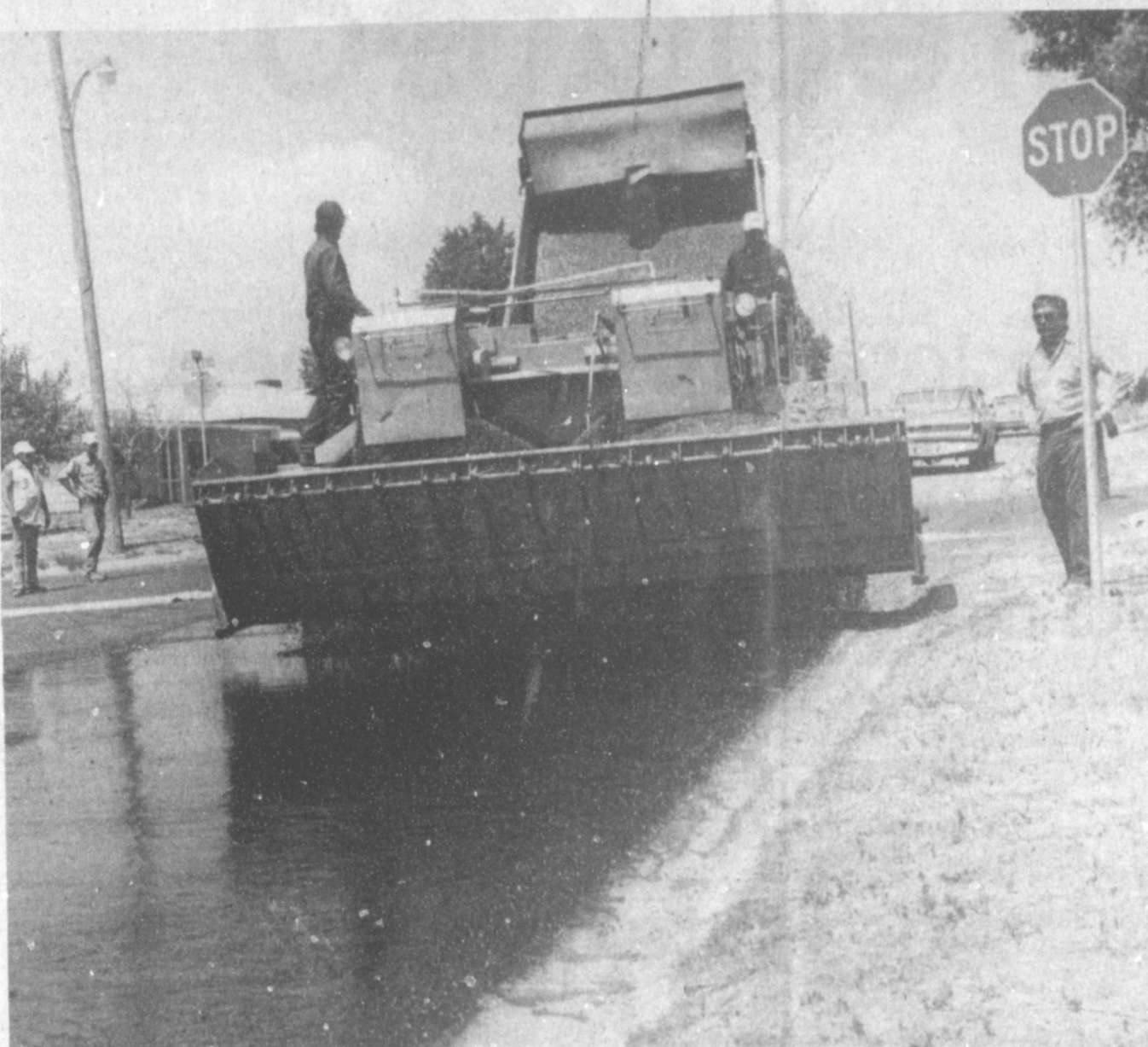
SEALCOATING GOING ON IN MULESHOE --Each summer, a certain number of streets are seal-coated in Muleshoe, and this summer is no exception. Hot asphalt and gravel are being put on a number of streets in the city, in a never-ending battle to keep the streets as much as possible, without potholes to have to try to drive over. Here, the paving contractors are laying a new seal coat on a city street. (Journal Photo)
