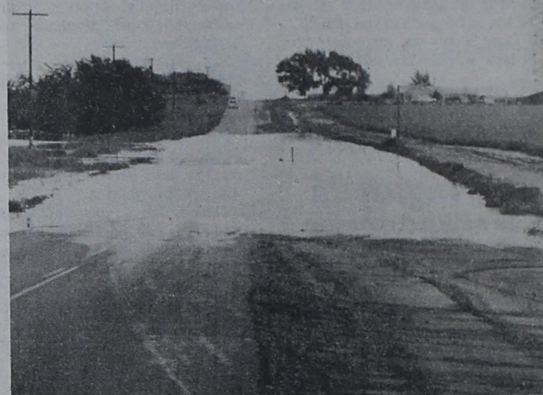
SPRUNG A LEAK... This west of Lazbuddie, which was covered in water from the recent rains. Shown is the highway FM 145
