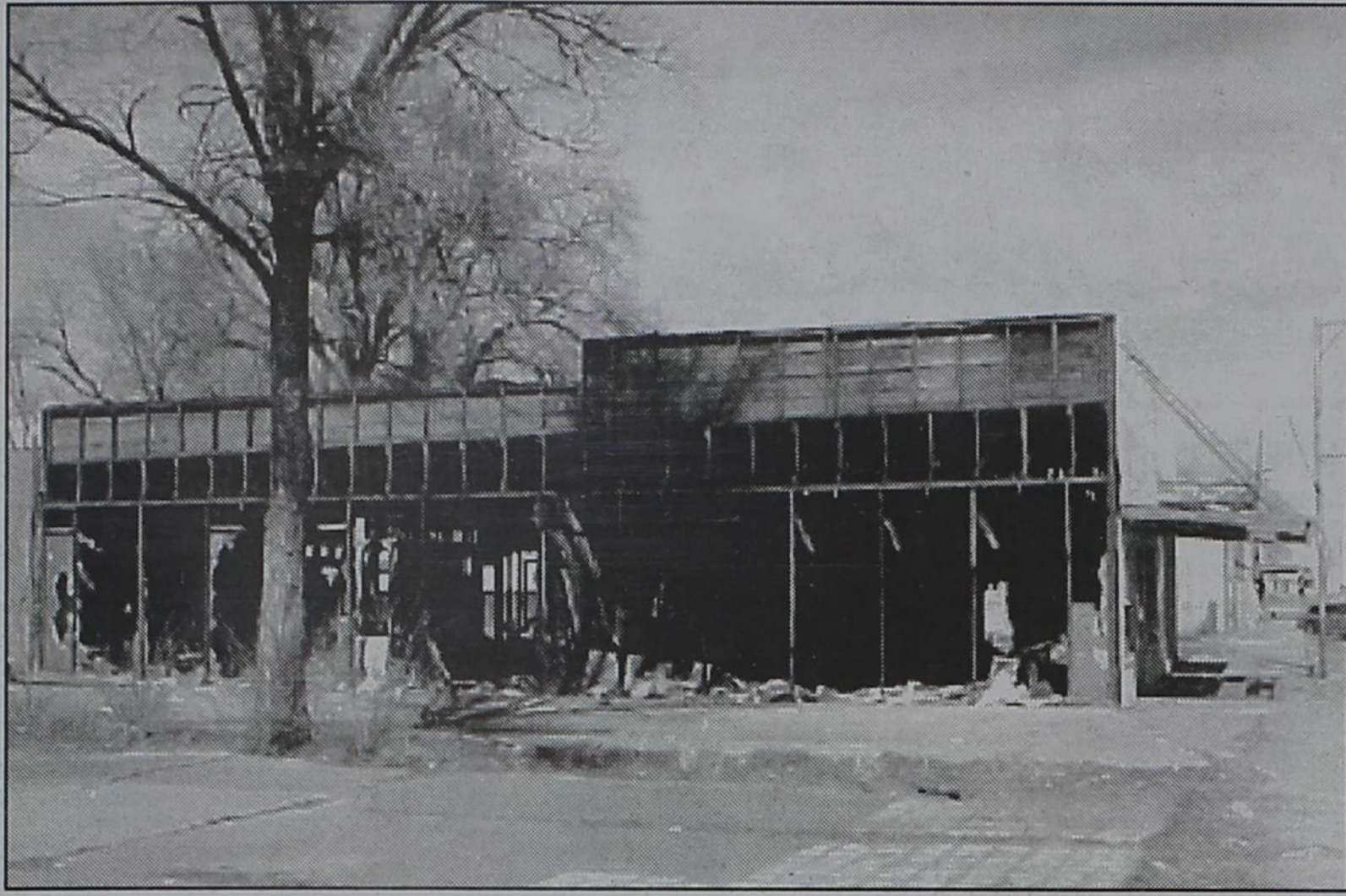
THIS OLD BUILDING on North Street is gone by now. It was in the process of being demolished last week. A fire farther down the block left North Street vacant except for the old hotel and a residence next door. ron carr photo
