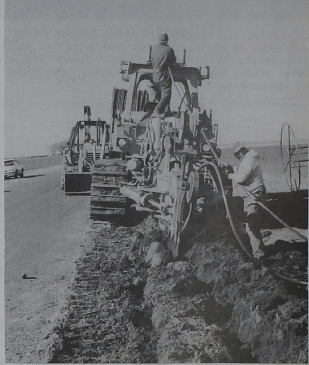
INSTALL CABLE.... Crew members from Brooks Construction Company, contractor for a cable-laying project for West Texas Rural Telephone Cooperative, are shown at work on installation of a stretch of cable that's part of the 40 miles of fiber-optic cable being buried by the cooperative in an ambitious upgrading project in Parmer, Deaf Smith and Castro counties. Upon completion of the project, all of WTRT's central offices in Parmer, Deaf Smith and Castro counties will be linked by fiber-optic cable. (WTRT Photos)
