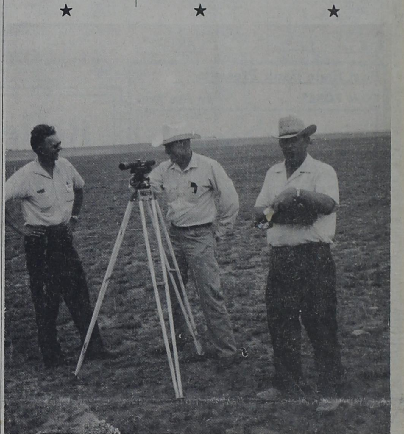
SURVEYING FOR NEW DAM --- Herb Evans discusses survey work on the proposed dam on Catfish Draw two miles north of Bovina with Al Lee of Hereford, at the instrument, and Ed Fry of Tulla, who is taking notes. Lee and Fry are members of the survey crew and Evans is head of the Soil Conservation Service in the county. The new dam will be located just downstream from Mustang Lake, a cattleman's landmark in the area for generations.
