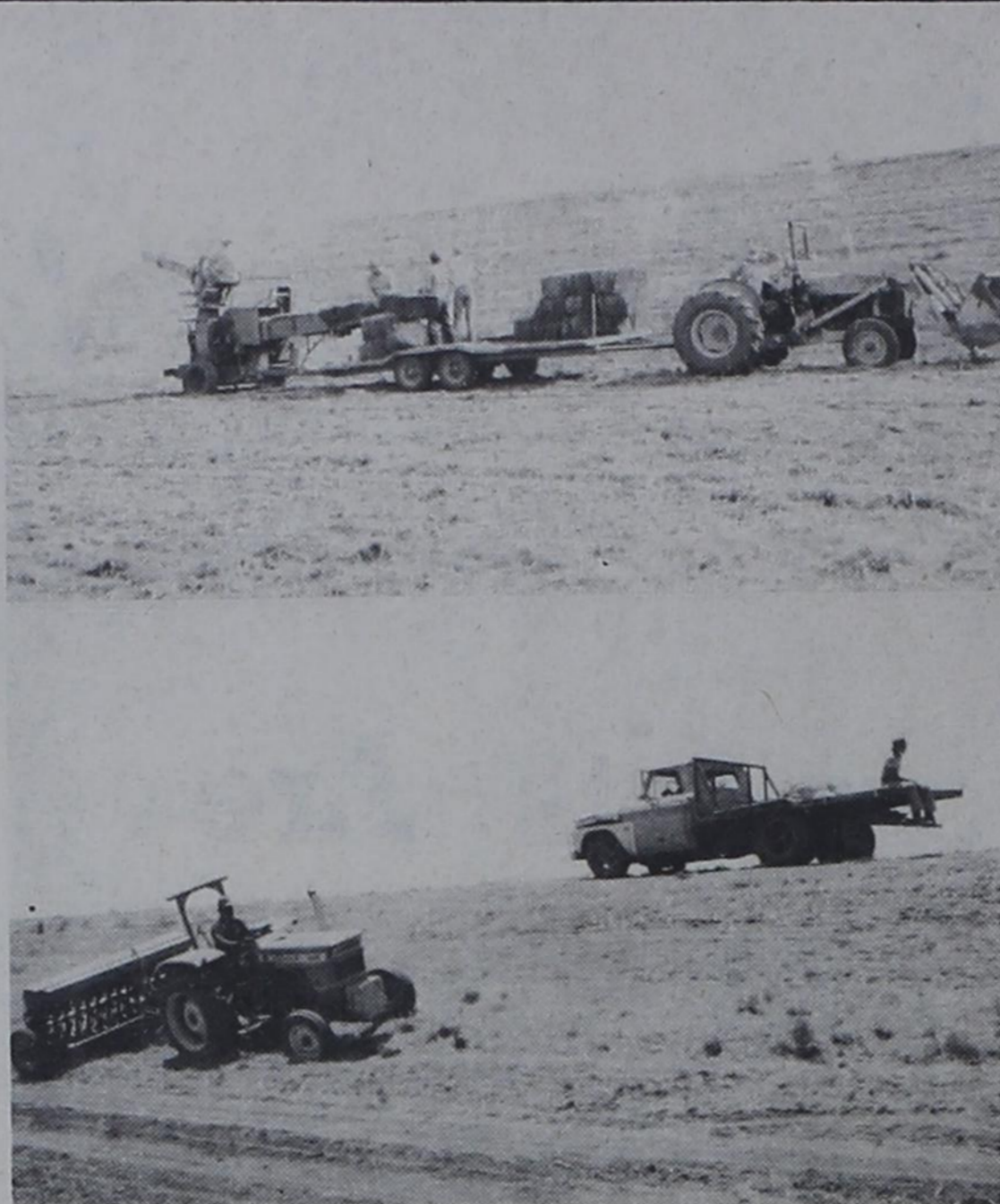
RESEEDING DAM.... Employees of the Bachmayer Company, which has been contracted to reseed grass on the Bovina Dam, in the top photo, are shown blowing prairie hay mulch on the dam as part of the
