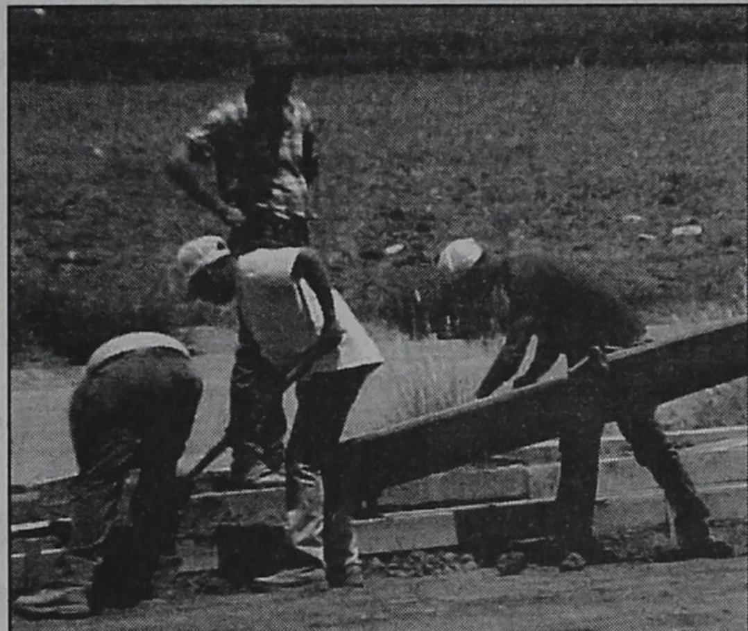
WORKERS FROM Ruben's A-1 Construction of Lubbock are installing the parking lot concrete curbing at Prairie Acres Heritage Estates. Shannon Cochran and Jeff Williams of T&S Concrete in Friona are shown delivering another load of concrete at the construction site. ron carr photo
