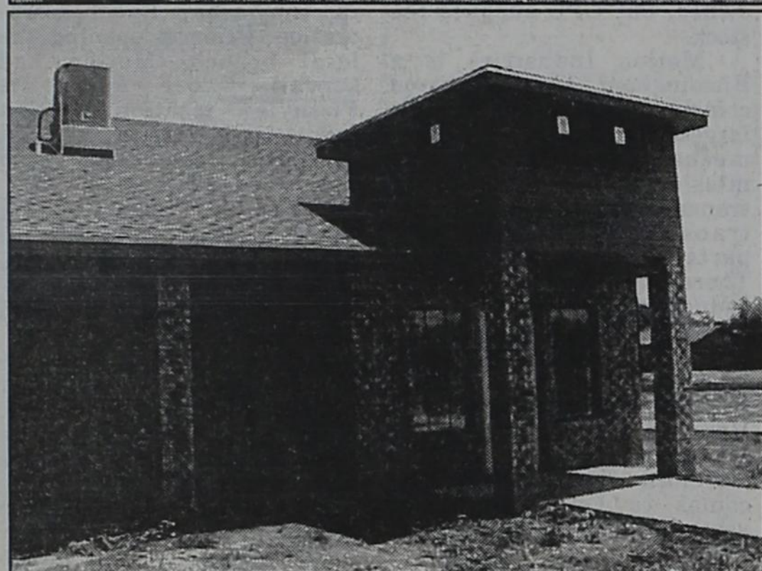
EXTERIOR VIEWS of Prairie Acres Heritage Estates. Construction continues on the assisted living facility. ron carr photos
