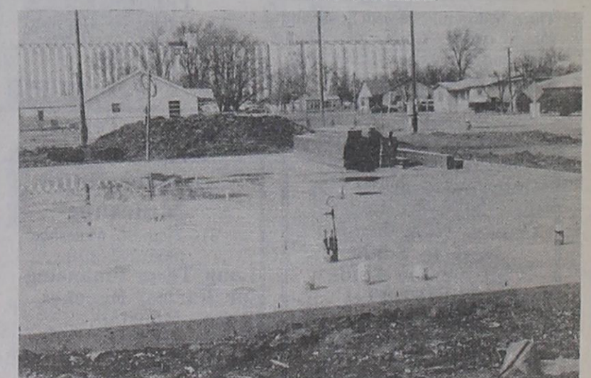
PIPES, WIRE, AND CONCRETE.... Workers are making progress on the new BISD administration building as long as the weather cooperates. The concrete slab is poured and plumbed. (ron carr photo)
