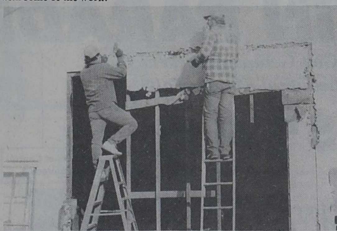
WORK BEGINS... Work is underway on renovating the former American Legion Hall on Third Street. The building will house Bovina Ambulance Service's equipment. Galen Hromas is in charge of the construction.
