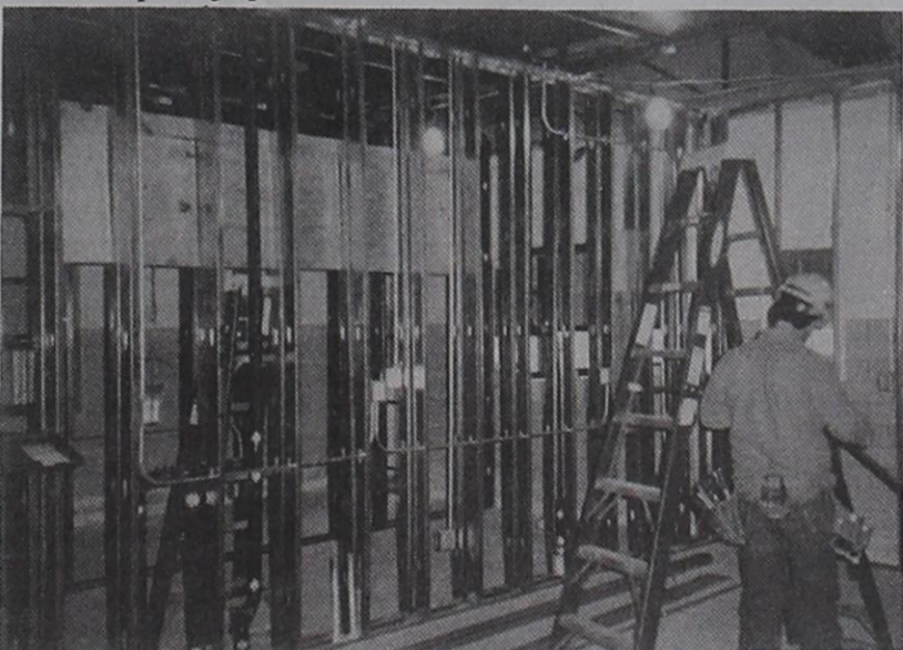
HELLO WALLS.... Work goes on in the cafeteria as workmen started building the walls during the past week. the cooler and freezer are to be installed in the next few days.
