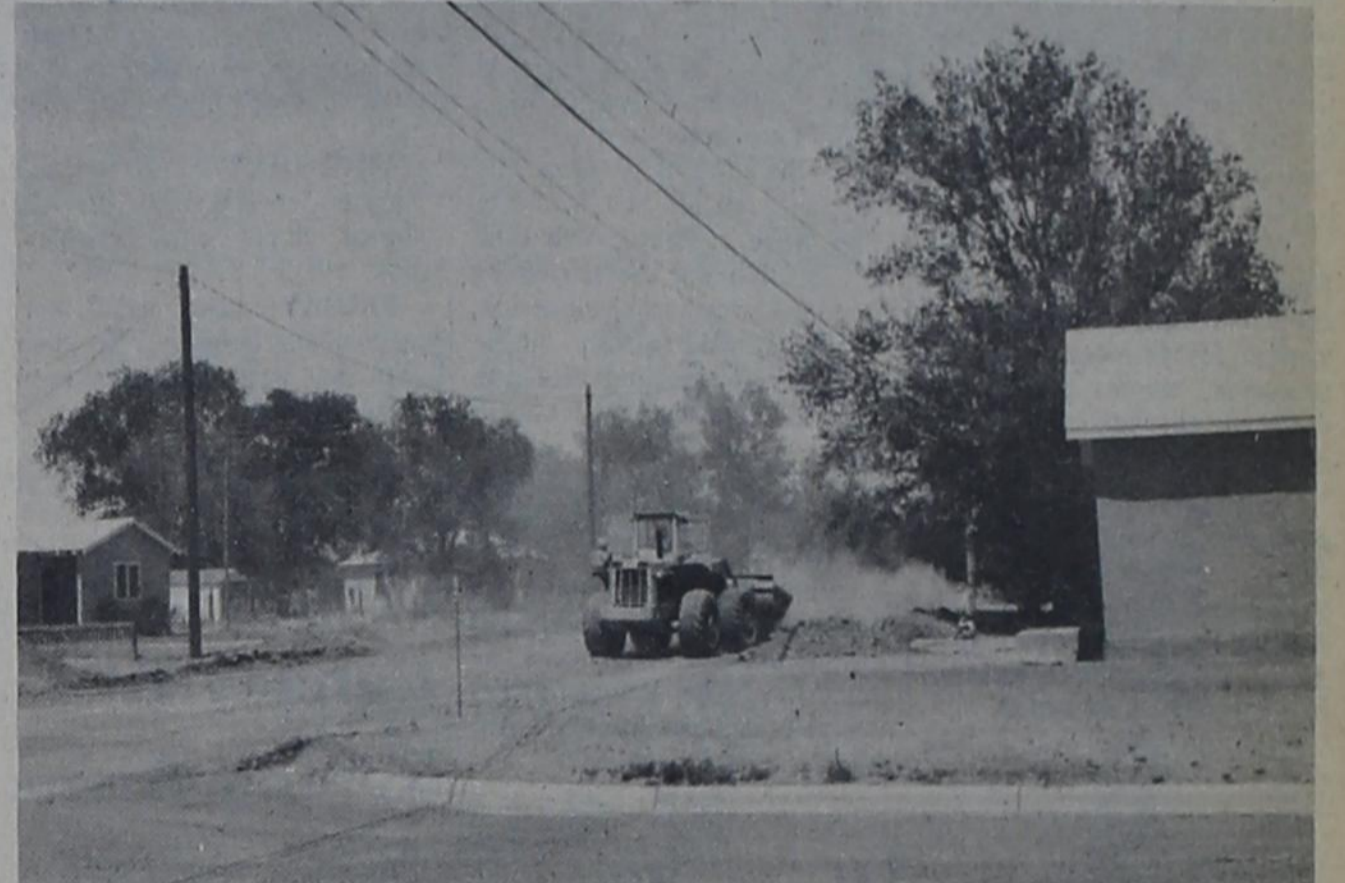
PAVING WORK BEGINS...The Jake Diel Construction Company began the initial phase of paving some 14 blocks in Bovina Monday morning. Scheduled for the improvements are portions of Fourth and
