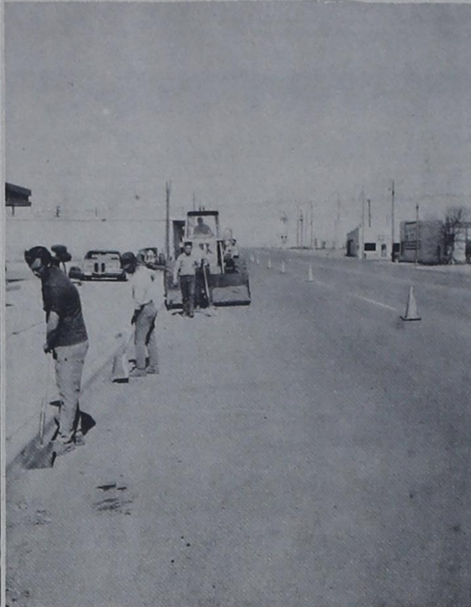
CLEAN-UP OPERATION --- Texas Highway Maintenance Department crews are shown working in Bovina recently cleaning sand and dirt from curbs on FM 1731 and Highways 86 and 60. From front to back, are Buck Page, Frank Galvan, Wilfred Sikes and Gene Bitner. Wayland Beavers is driving the loader.
