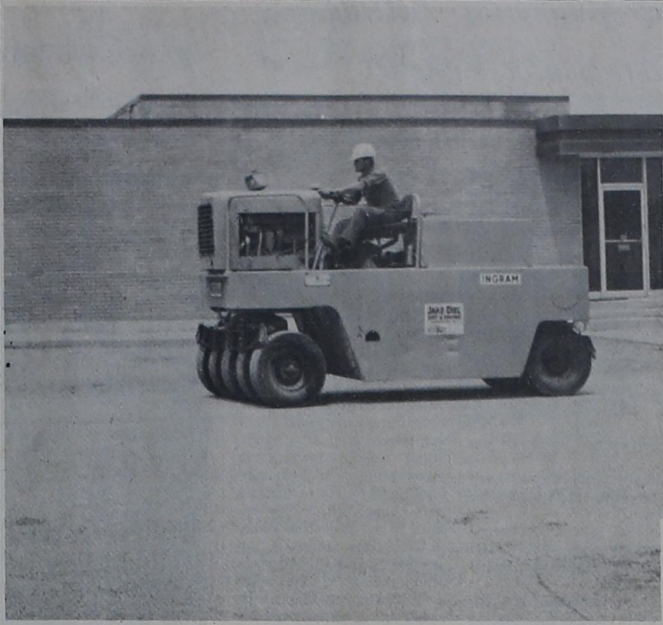
COMPLETE REPAIRS.... A workman from the Jake Diel Construction Company puts the finishing touches on Avenue A between First State Bank of Bovina and Allsups 7-11 Monday afternoon as 24 blocks of seal coating were
