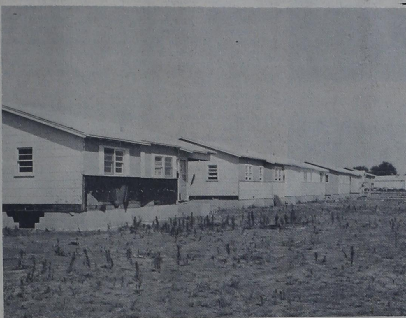
WORK PROGRESSES --- Nearly half of the houses scheduled to be moved here from Amarillo are on their foundations in Eastview Addition. Remodeling the houses is underway. A total of 26 are included in the project, which will be sold to prospective workers of Missouri Beef Packers who will move here from South Texas.
