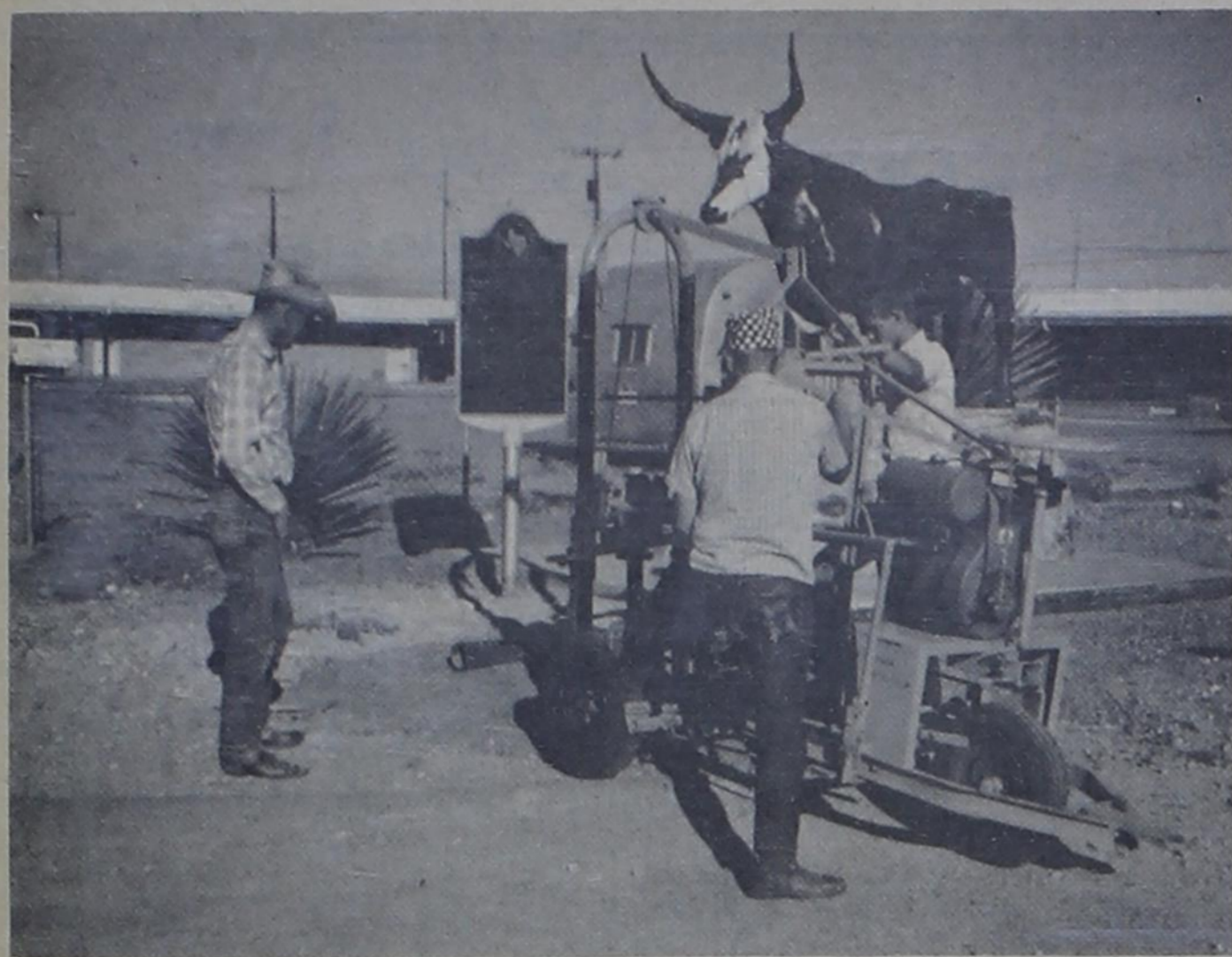
DON'T FENCE ME IN --- Contrary to imagined wishes of the early day cattle that roamed the open grasslands around Bovina, a fence is being constructed around the Bovina Bull by the State Highway Department on Highway 60. Both the statue and the historical marker tell the story of Bovina when it was a famous cattle-shipping point on the Santa Fe railroad. (Photo Courtesy Weldon Moody)
