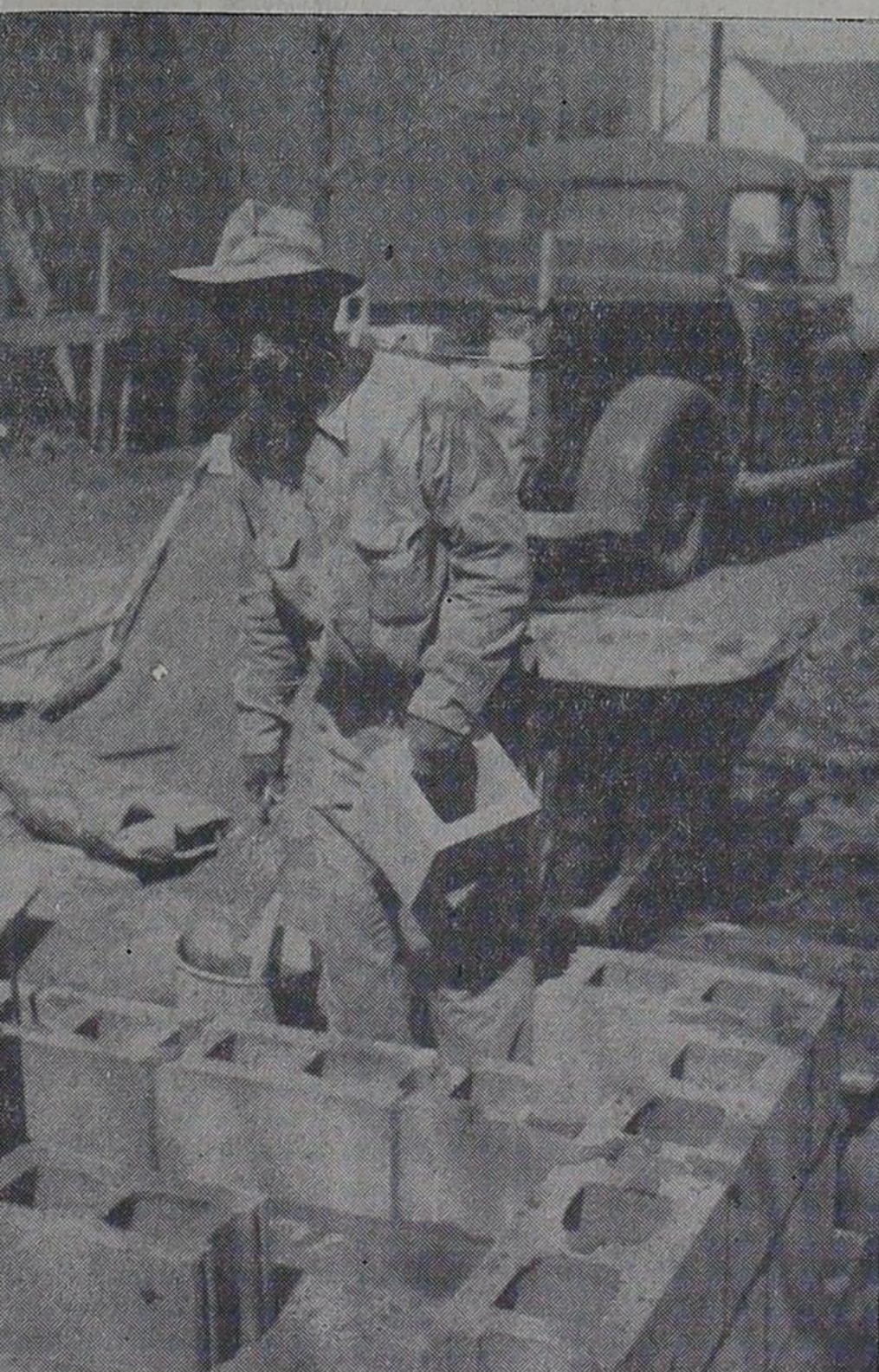
ADDITION TO CITY HALL — R. L. (Lum) Edwards is building the walls for the city's new warehouse which is scheduled to be completed within 20 days. The building which is to be 24 feet by 28 feet in size, is being built behind the city hall. It will be used to store city machinery and equipment. Approximate cost will be $1700, Henry Minter, city secretary, says.
