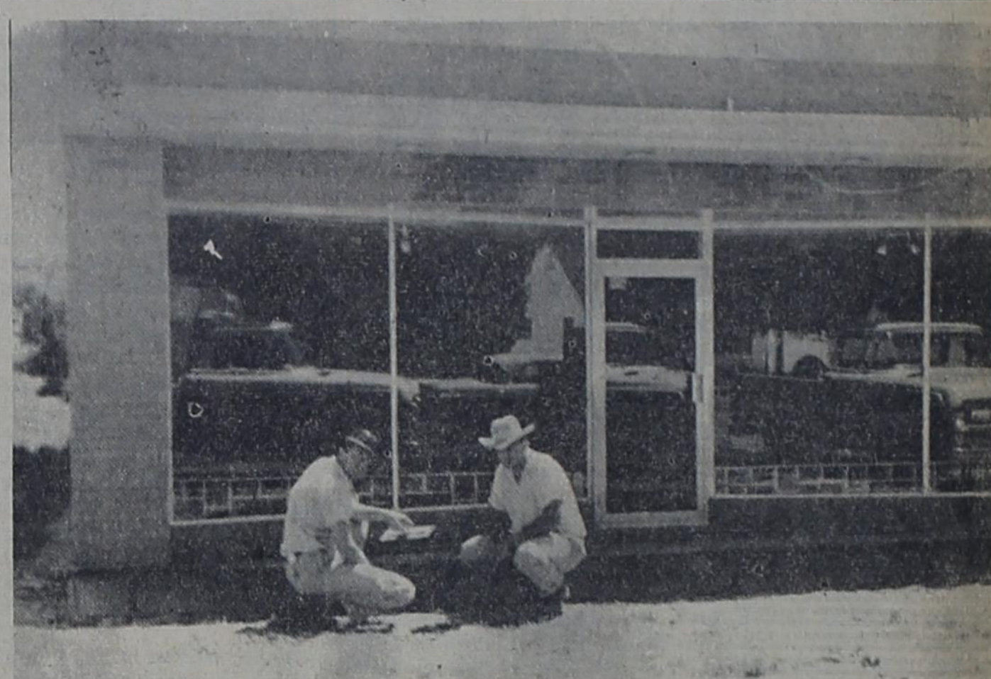
FINISHING TOUCHES--Henry Minter, left, and H. D. Turner put the finishing touches to cement in front of Mary Marr Shop that will open soon. Mary Turner and Margaret Minter will be operators of the shop that will handle ladies apparel. Minter and Turner constructed the building for their wives' business. It is located on Third Street. The ladies hope to open the shop August 1.
