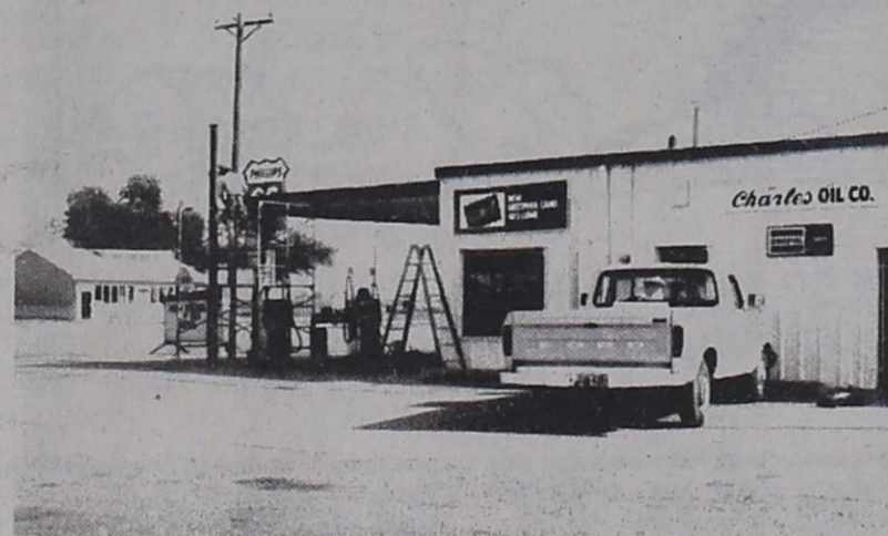
PHILLIPS MAKES CHANGE....Charles Oil Company is getting a new facial as work continues on the canopy at their building on Highway 60.
