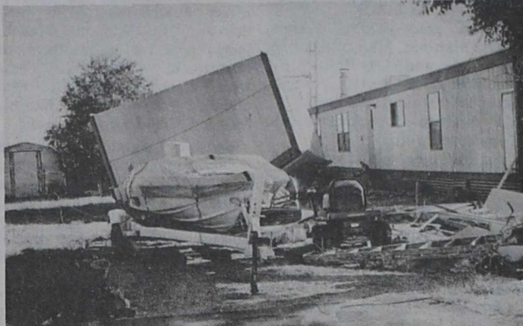
GARAGE DAMAGED... The garage at the Don Hatley home, three miles south of Bovina was badly damaged after a storm swept the area last Friday. The cloud was thought to be a tornado that didn't completely touch down.
