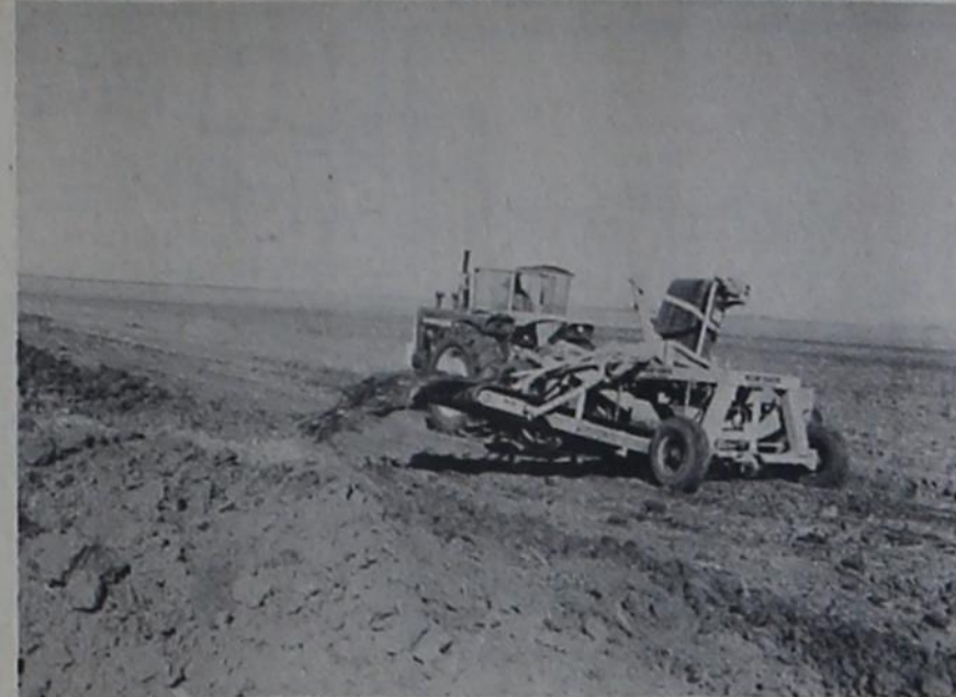
TERRACE CONSTRUCTION --- Parallel terraces, such as this one in the construction stage using a two-way belt machine, are being built in Parmer County under Great Plains Conservation Program and are designed and laid out by SCS technicians at the Friona work unit. Terraces such as these can be built through the cost share plan through the Parmer County Soil Conservation Service.
