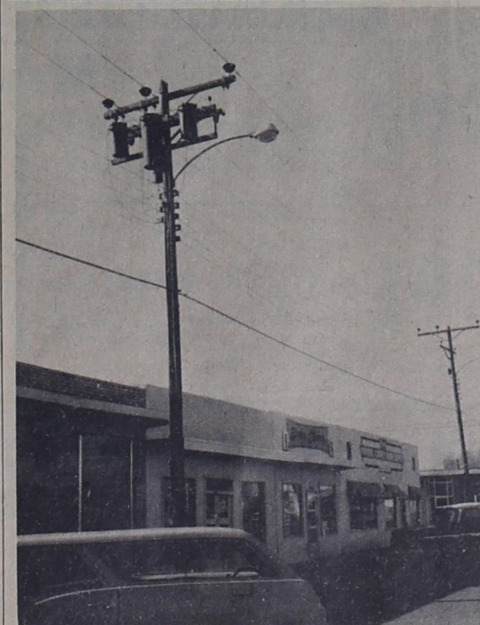
BEFORE -- Once Bovina's electrical power ran through these lines on Main Street, but with the relocating of the lines by Southwestern Public Service Company, the transformers and lines were no longer needed. The project to "clean up" the poles was started several weeks ago.
