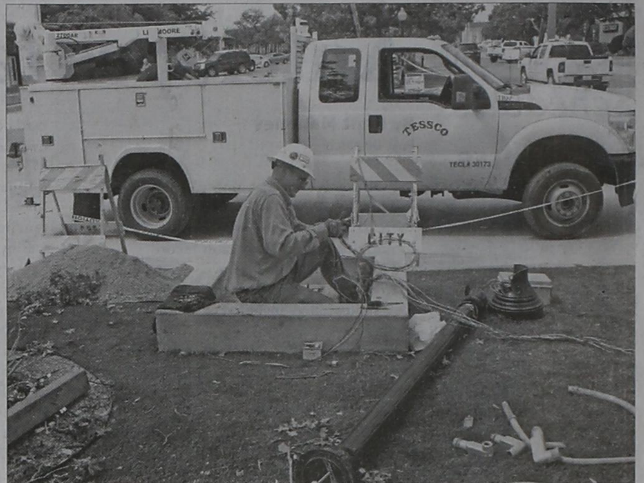
Dustin Buzbee, of Levelland, begins repairs on the electrical on Main Street after an 18-wheeler performing a U-turn knocked it down. Buzbee was hoping to have the repairs finished by the end of the week, but was having problems finding a match to the light globe that sits on top of the street light.
