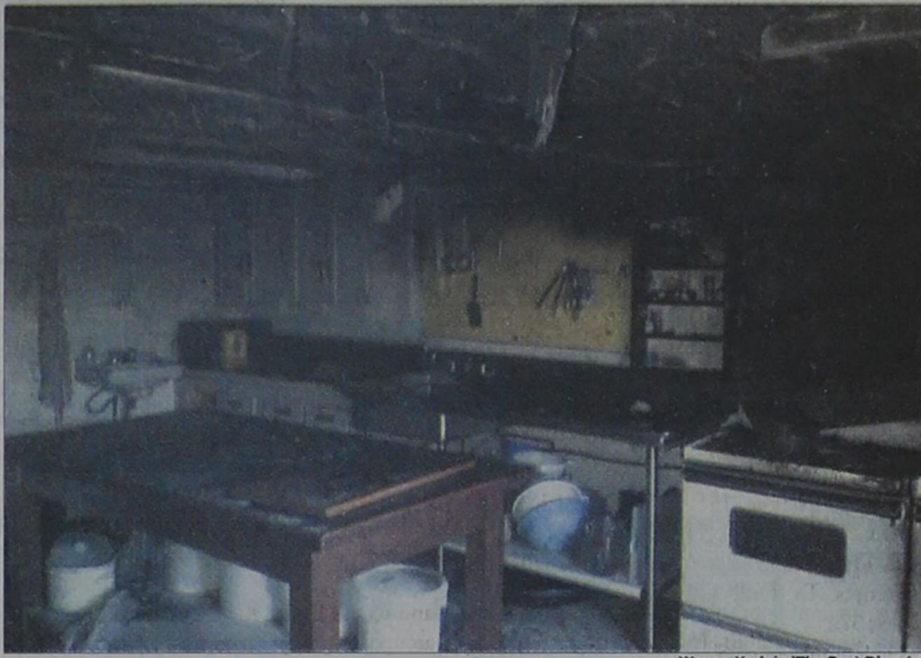
Top: Post volunteer firefighters work Tuesday evening to clear smoke from the historic Garza Hotel in downtown Post after a grease fire broke out in the kitchen. Bottom: In this photo, provided by sheriff's officials the fire has burned the ceiling and surrounding areas.
