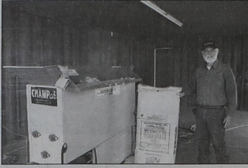
Mike McGuire and Western Fibers retrofit houses across the state with new insulation manufactured in Hollis. This house is northeast of town.
