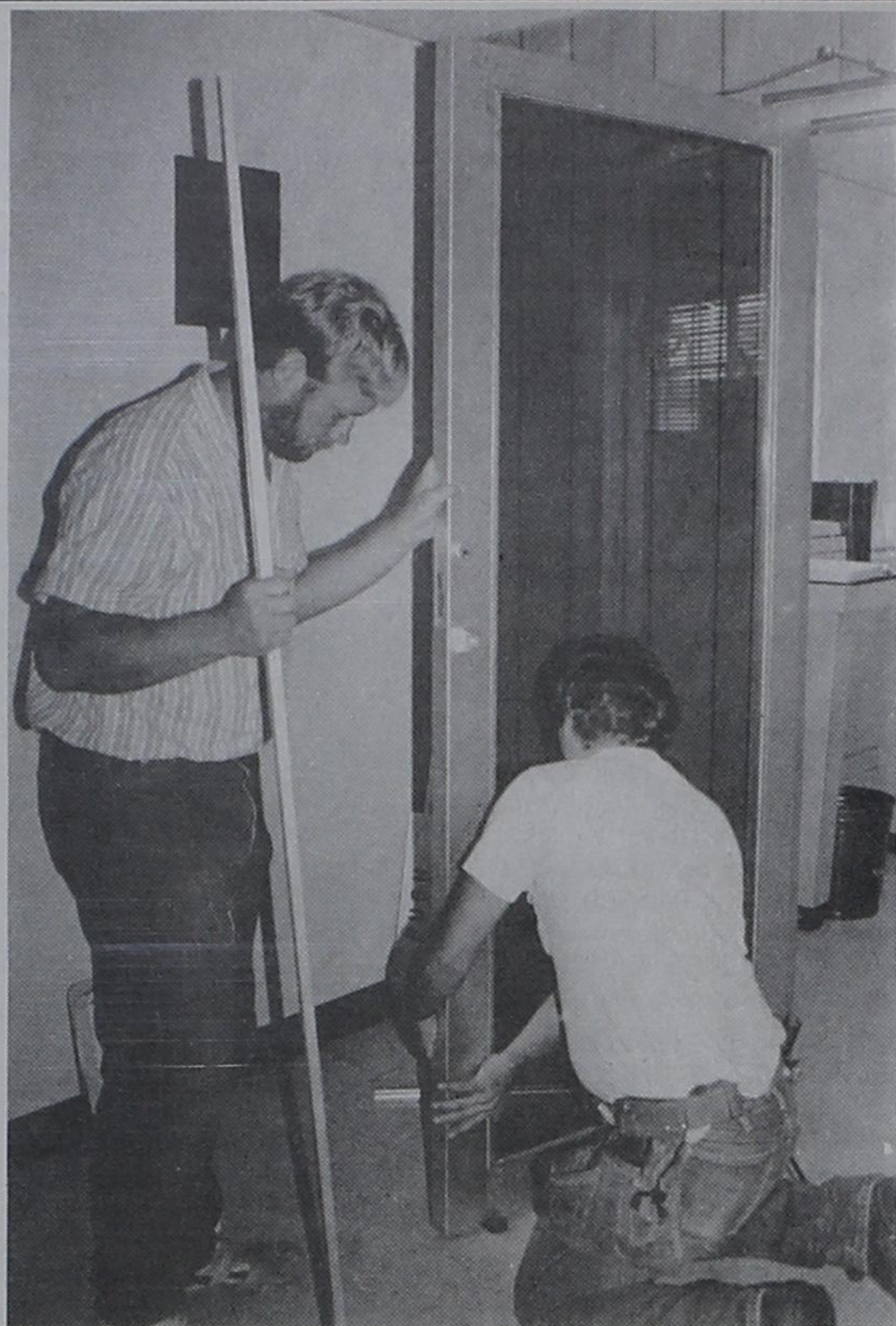
NEW DOOR...Repair workers from Clovis Glass Company replaced the glass in the door leading into the post office business counter, which was broken by burglars to gain access into the work area where some items were taken early Monday morning.
