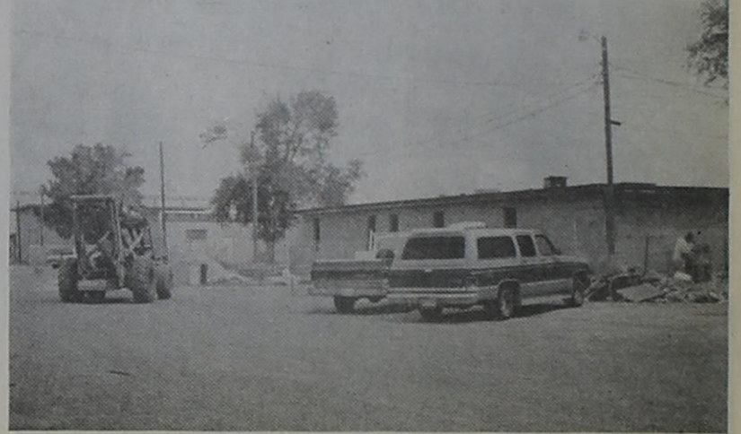
NEW CONSTRUCTION....The Bovina ISD is expanding its facilities to include five new classrooms and an expanded computer lab. The new rooms will be used for English as a second language, Special Education and classrooms for high school students. Completion is expected by September 1.
