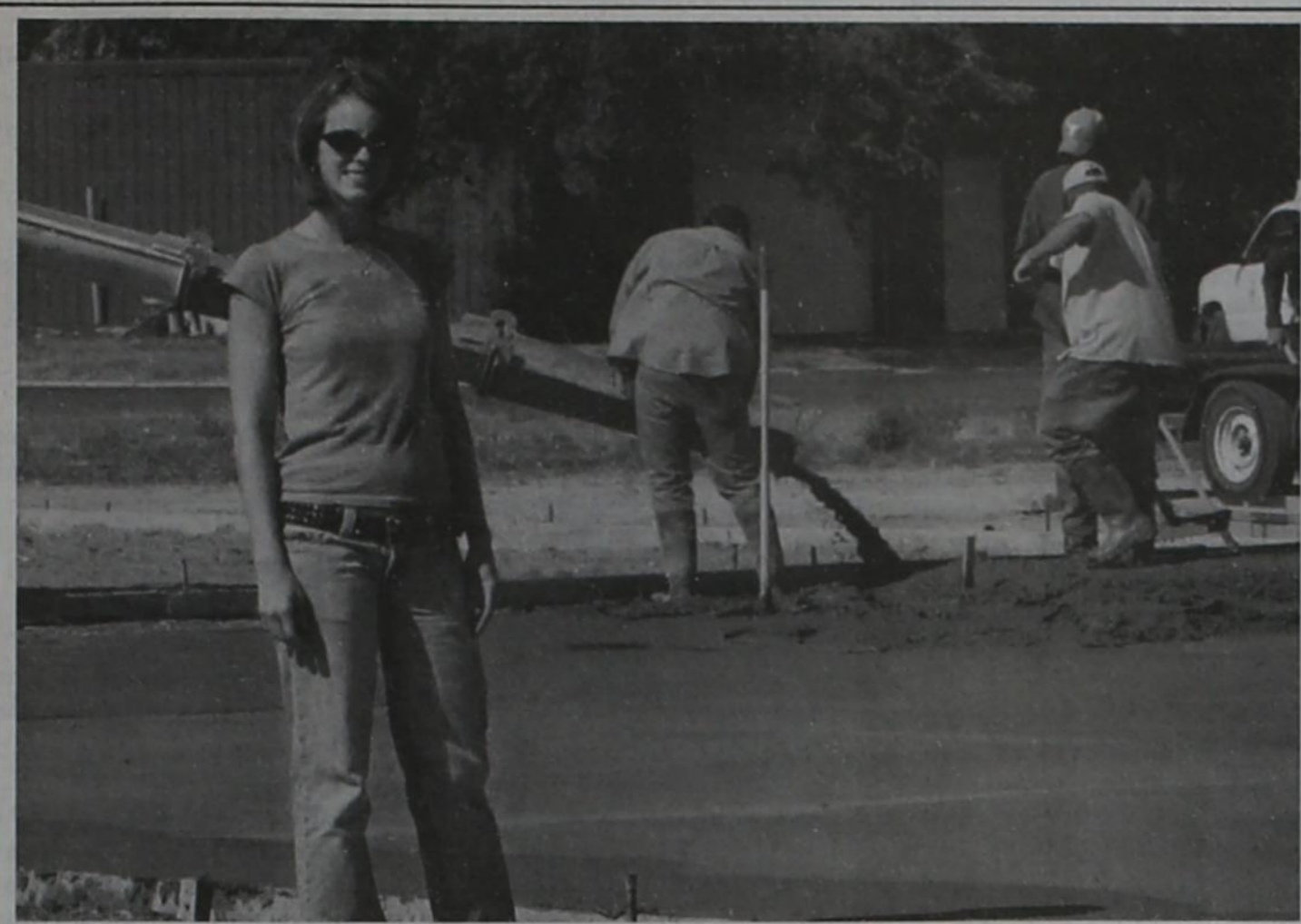
Standing in front of the newly poured cement at the corner of 8th Street and South Ave I, Krishna Bush happily watches the construction progress of the Post Skate Park. (Staff photo by Merika Strivens)
