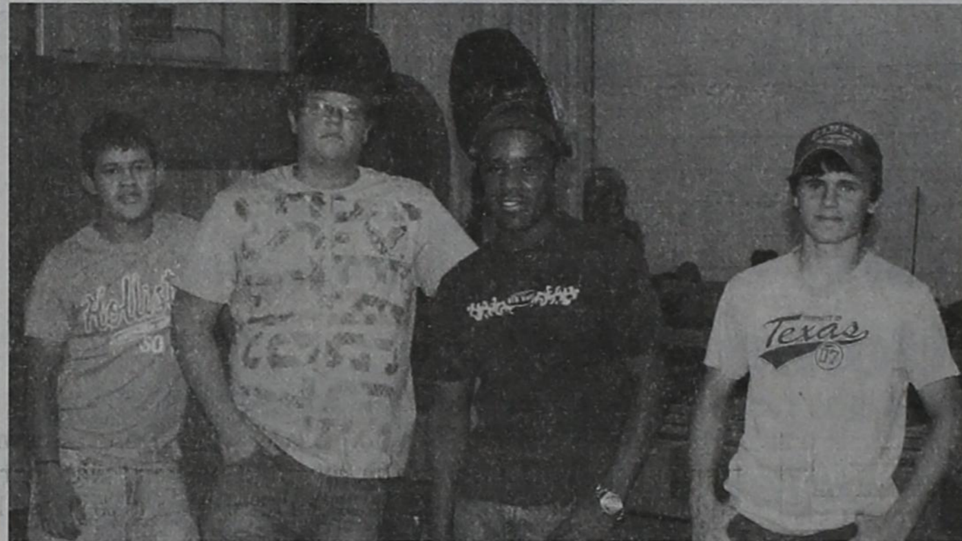
Nick Rodriguez (left to right), Heath Palmer, MJ Wynne and Trent Laurence helped put a metal floor in a 32 foot flatbed gooseneck trailer. They are enrolled in Ag Mechanics classes at PHS. (Photo by Merika Strivens)
