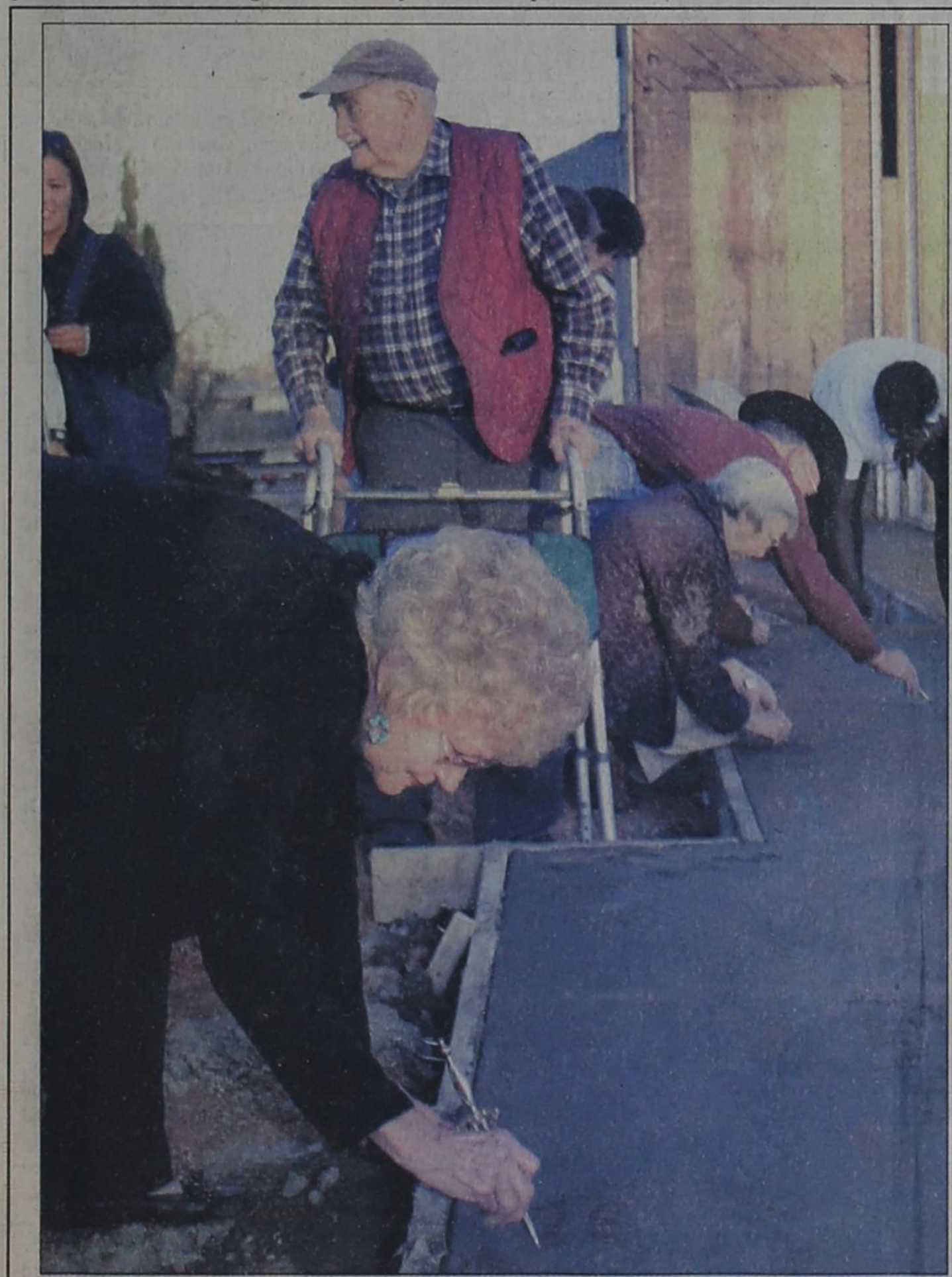
Caprock Cultural Association board member Glenda Morrow (front) signs her name on the concrete slab of the Heritage Center during last Thursday's ceremony at the construction site next to the Garza Historical Museum. Morrow was joined by other CCA donors and friends of the Heritage House project. The special event included a construction update by Don Collier and a champagne toast. Collier reported that the Heritage House should be completed during the month of May. Others participating above are Lewis Earl, Jimella Simpson, and Pat Cruse (far right).
