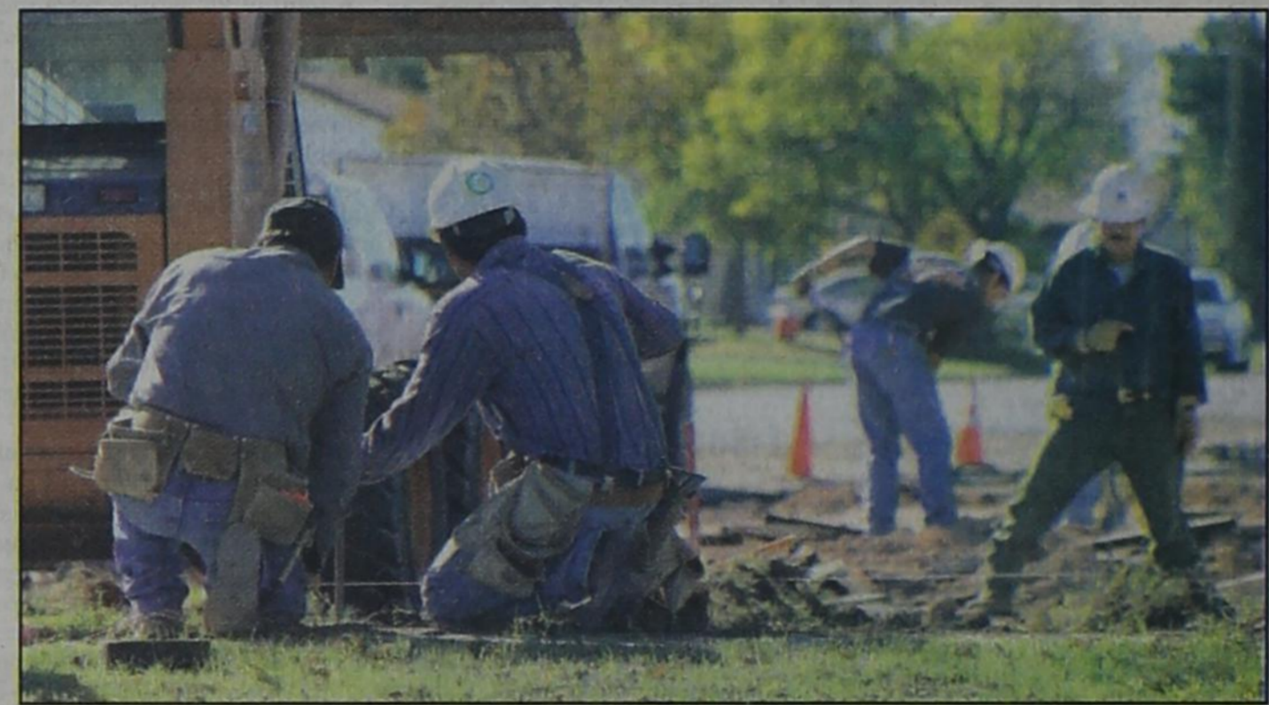
The crew of Joe Marts Construction are shown building a new parking area last Thursday on the east side of Post Elementary. According to Post ISD Superintendent Marlin Marcum the cafeteria construction work is on schedule and set for completion during the upcoming Christmas break and will be ready for use at the start of the spring semester. (Staff photo by Tim Burnett)
