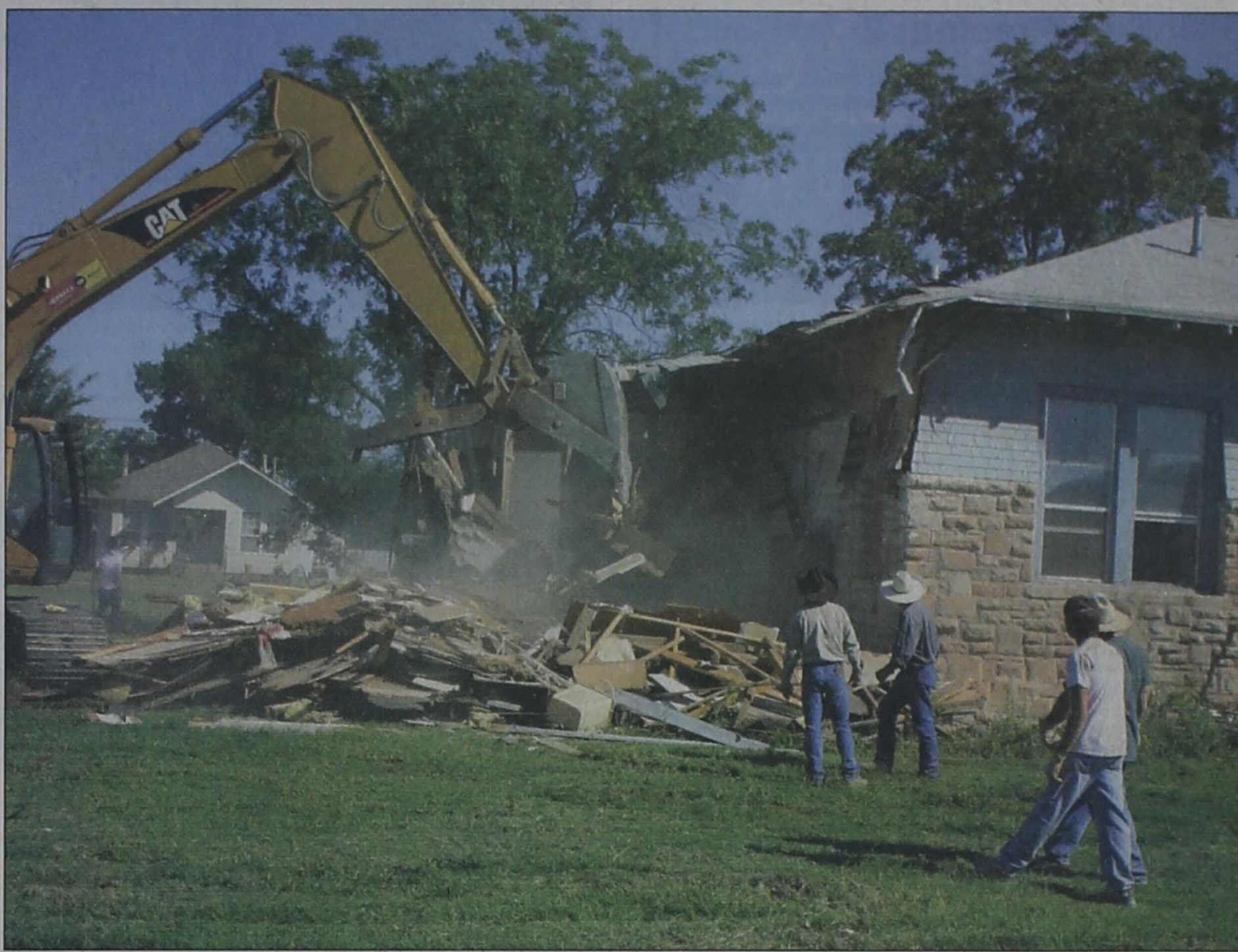
A piece of Post history came down recently with the demolition of one of the earliest houses built when C.W. Post founded Post City. The house was located on North Avenue I near the corner of East 10th Street.
