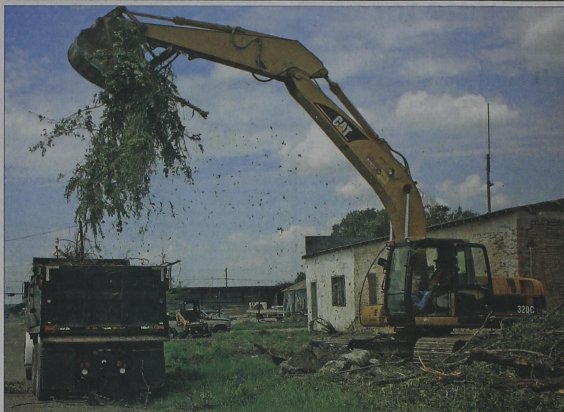
Contract work began last week to demolish two old buildings on Avenue I at the corner of 8th Street in preparation for City of Post plans for a parking lot. The buildings were the subject of condemnation proceedings in district court action.
