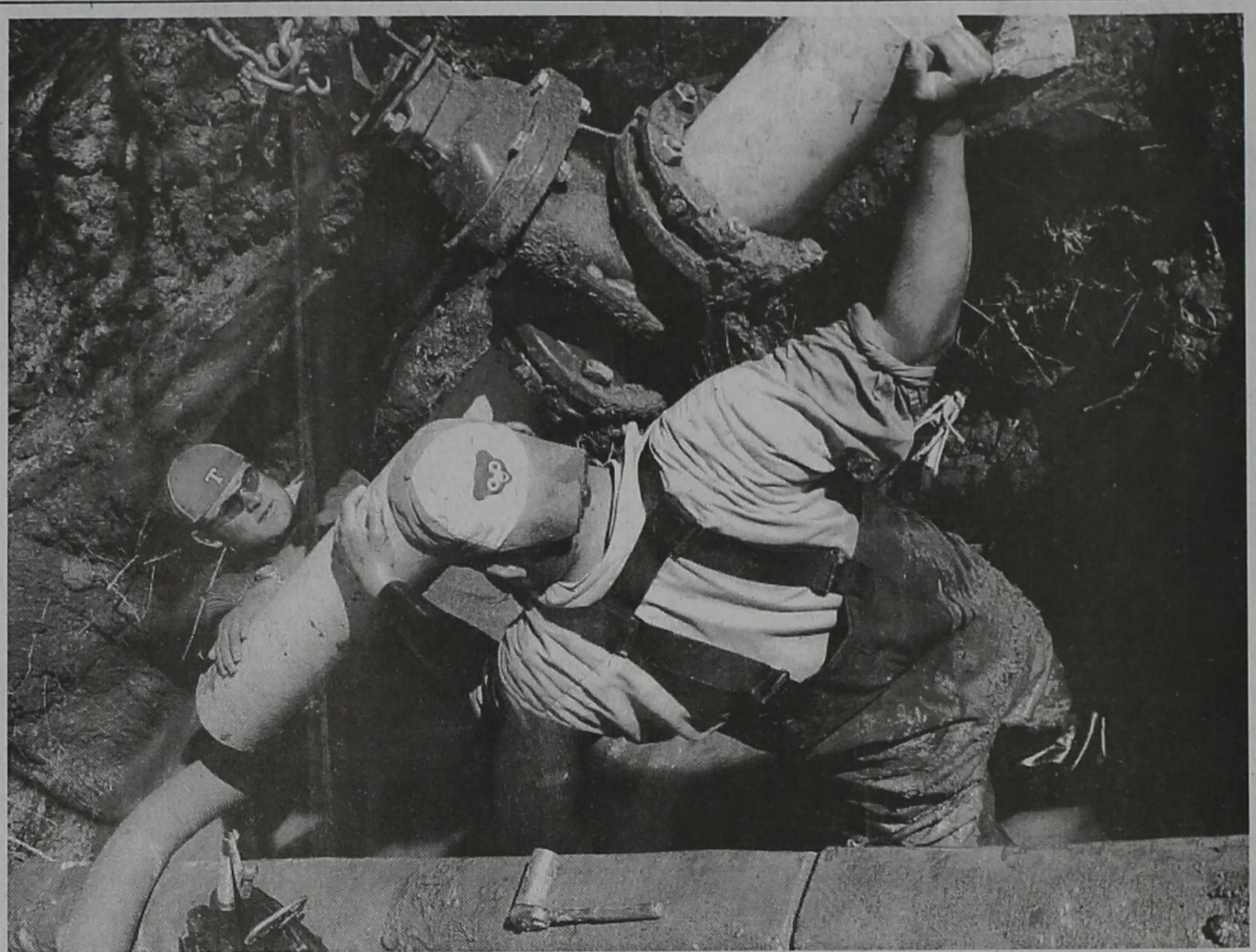
City employees repairing a six inch water main leak on Avenue M between 11th and 12th street are (left to right) Bryan Looney and Lazaro Moreno. Also on the site were Curtis Martin, Johnny Torres, Owen Gilbert and Frank Flores. The team labored into the afternoon last Wednesday, January 18, in waist deep standing water, and carefully negotiated the job near an exposed gas line. (Staff photo by Tim Burnett)
