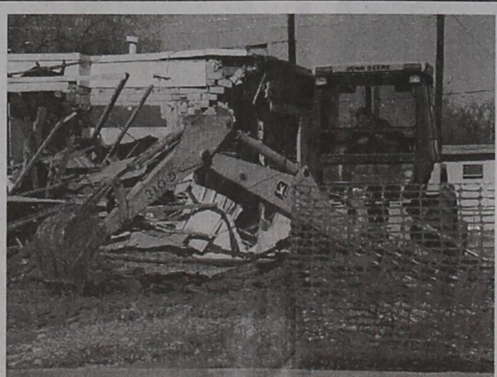
Jim Wagner, from Lubbock, operates the back hole while pulling the former unattended gas station on 10th Street and Broadway for New Mexico based "Three T" Properties. (Staff photo by Tim Burnett)
